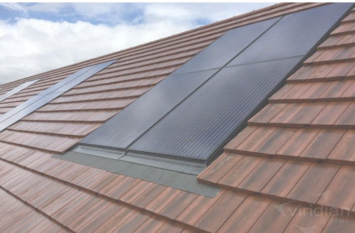
'IN-ROOF' SOLAR PANELS
