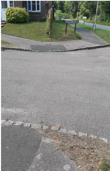
Figure 2: Existing alignment and upstand issues at crossing point.
