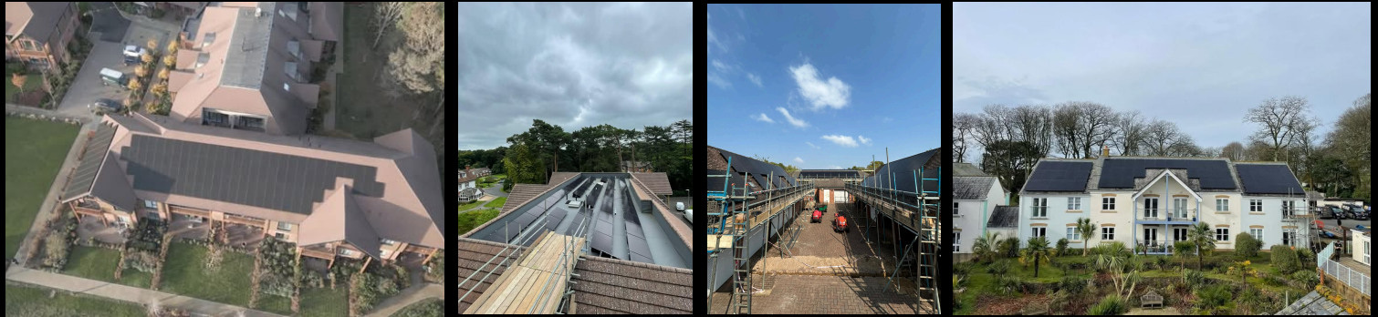
230kWp Project - Chailey Heritage Foundation
