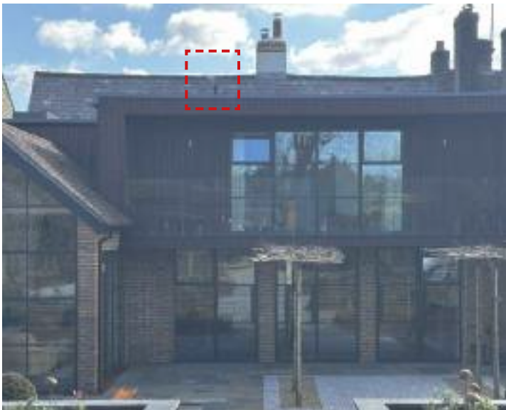
Recent photograph capturing the new boiler flue
