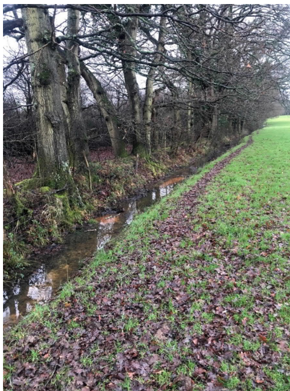
Image 2: Drainage ditch to the north of substation. Waterlogged after prolonged heavy rainfall.
