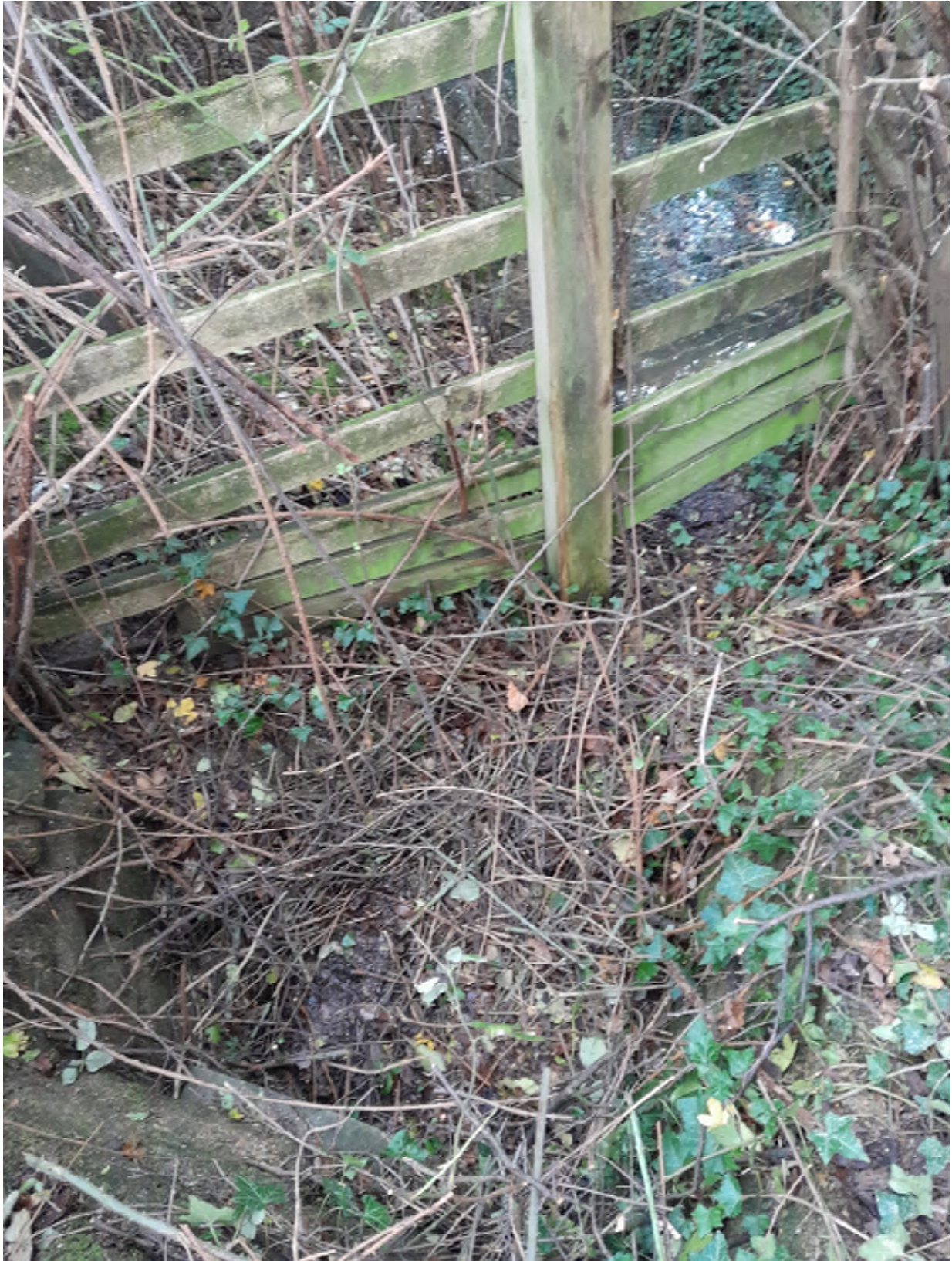
A2300 Culvert entrance and upstream section of ditch part full with water beyond fence – November 2022
