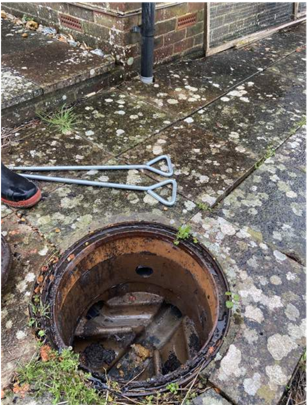
MH02 Inlet from MH01 Inlet from rainwater downpipe from main roof of dwelling
