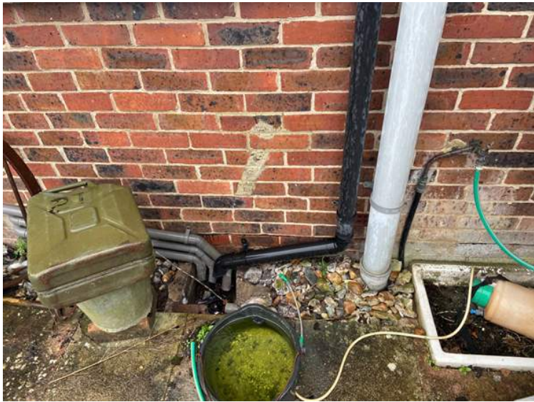
G01 / SVP01 Rear elevation SVP to bathroom Combined gully pot taking bathroom greywater and rainwater downpipe from main roof of dwelling
