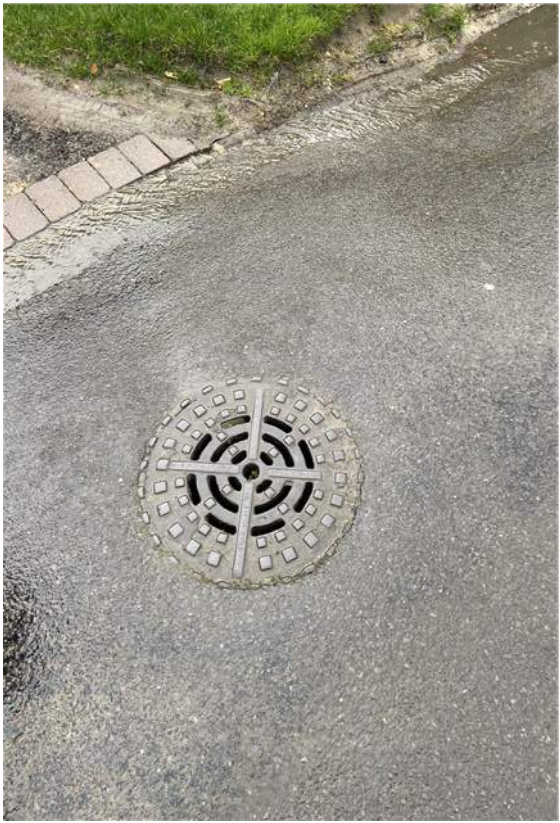
MH05 Grated public sewer manhole cover in College Lane
