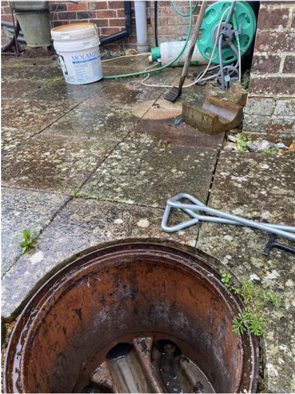
MH01 Manhole chamber collecting G01 and SVP01
