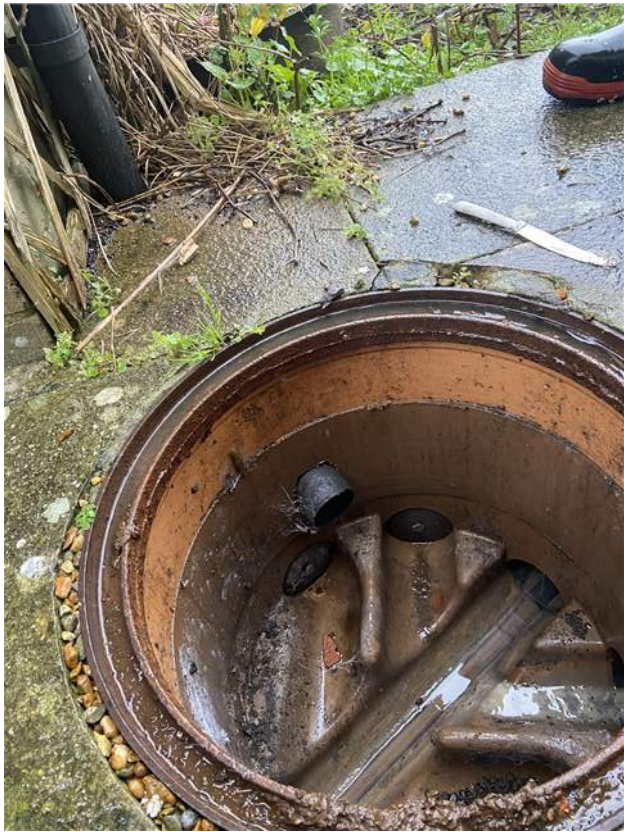
MH03 Inlet from MH02 Inlet from G02 Inlet from downpipe from garage
