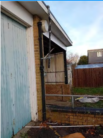
Suspected (decommissioned) vent pipe to underground tanks.
