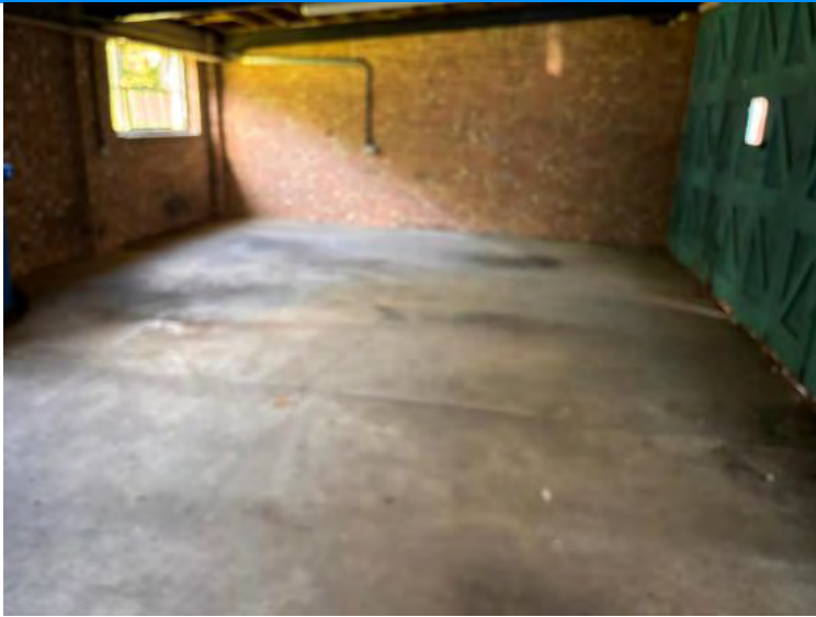
Inside the garage, with evidence of hydrocarbon staining
