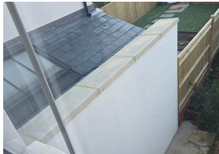
Fig. 5: Photograph of neighbouring extension (No.142) with white rendered finish.
