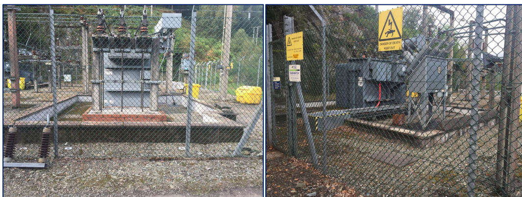
Figure 6: Typical bunding at substations
