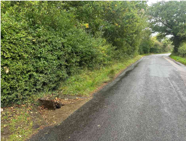
1, 0.00 m Start node, gully, reference: RG
