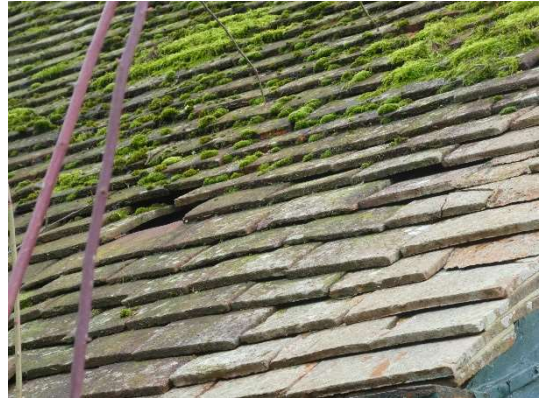
Photograph 8: A few slipped roof tiles upon the western roof pitch.
