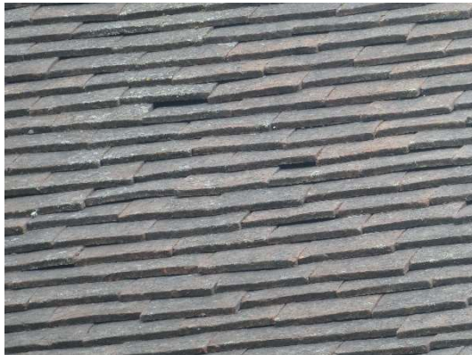
Photograph 3: Occasional gaps were present under roof tiles.
