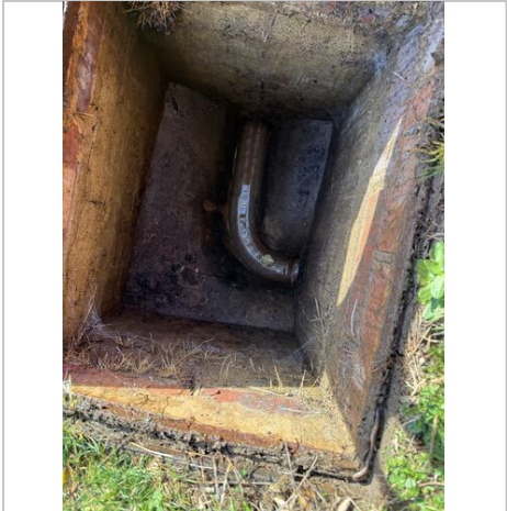
Manhole leaving 48 02 Mar 2026 09:55
