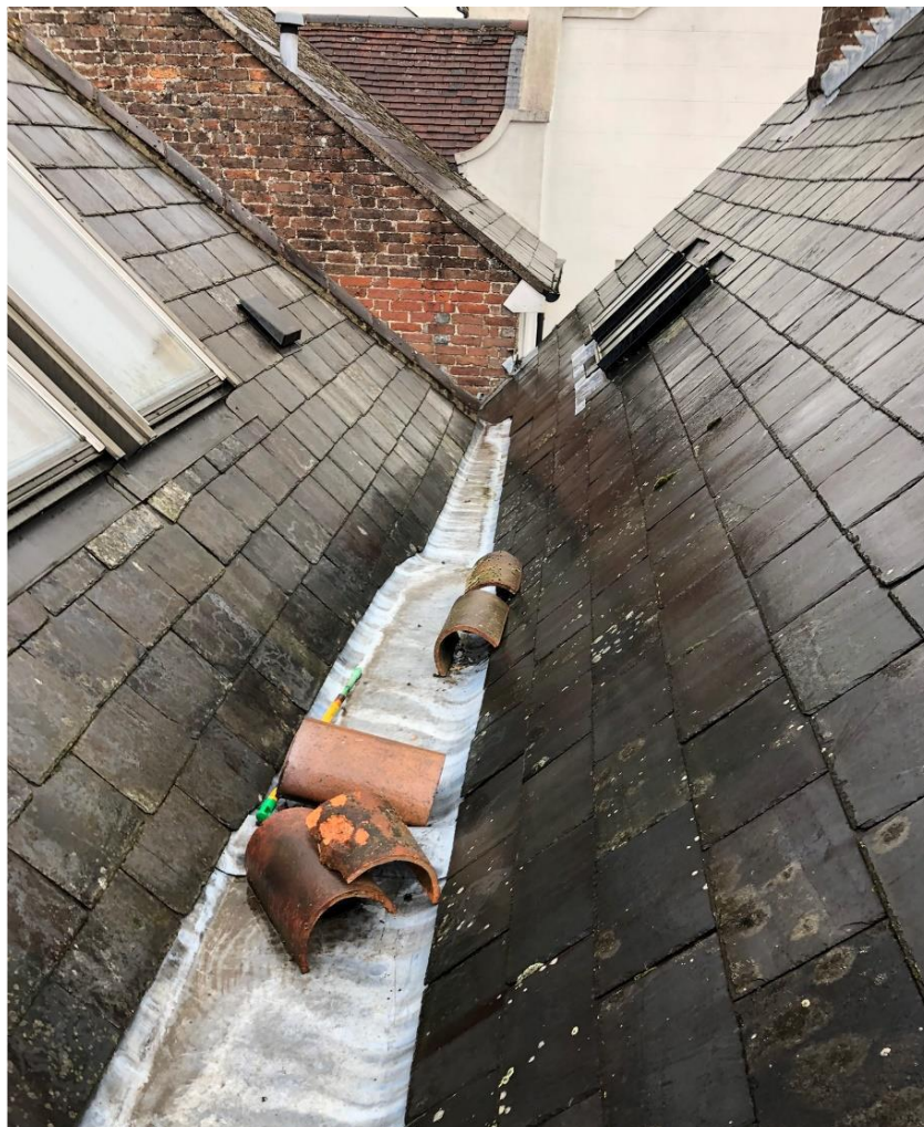
Figure 30: the rear roof slope to the original 15 th century building contained no less than 5 rooflights prior to their removal and slating over as part of the implemented scheme. Source: Gould Baxter Survey (October 2022)
