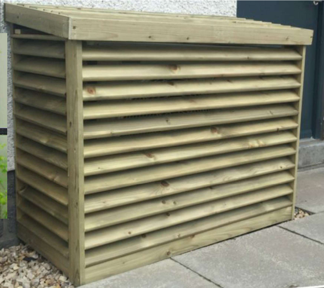
Air Source Heat Pump louvered wooden guard
