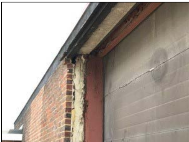
Photograph 4. An example of gap in masonry of the industrial building affording potential access into cavity wall.
