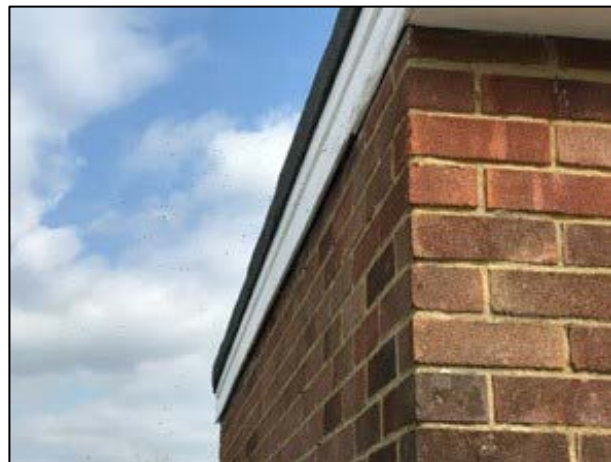
Photograph 7. A gap behind the barge board on the extension of the industrial unit potentially affording access to a void space between roof and ceiling.
