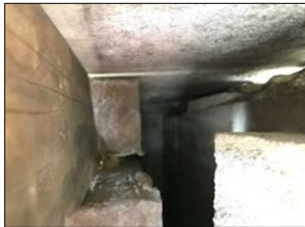
Photograph 5. A photograph of inside the industrial building's cavity wall (taken using an endoscope).
