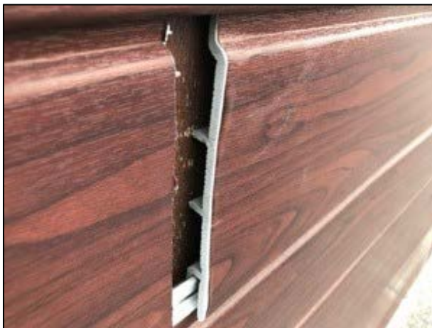
Photograph 6. A gap in plastic cladding on front elevation of the industrial building.
