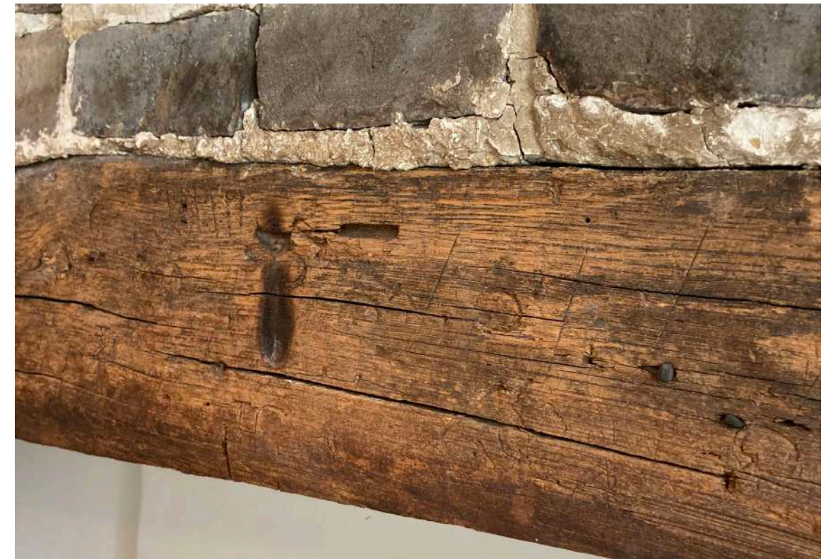
Evidence of burnmark to inglenook bressummer beam
