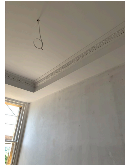
Example of ventilation dropped ceiling with cornicing
