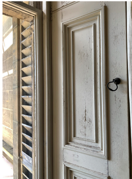
Example of timber shutter requiring restoration
