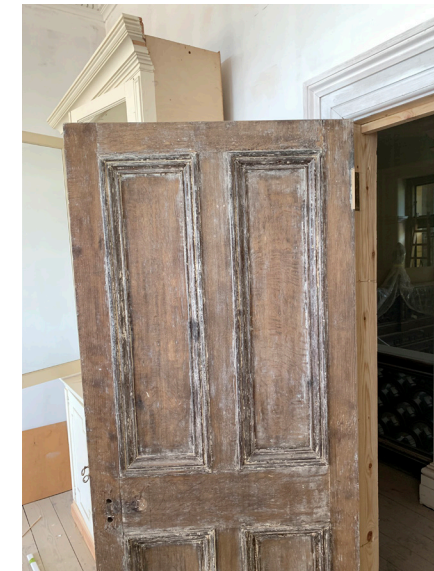
Example of door restoration and decoration required
