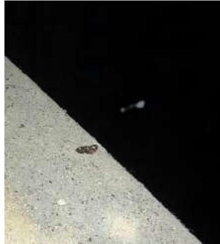
Fig. 6 – bat dropping on ceiling timber
