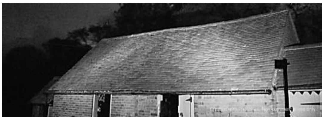
Fig. 14 – IR camera view of outbuilding roof, Survey 1
