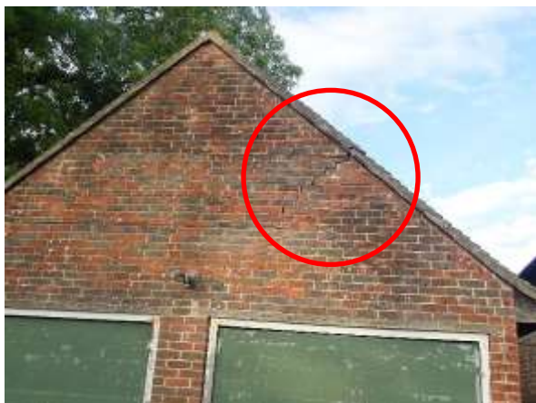
Fig. 12 – Crack in west end wall of garage
