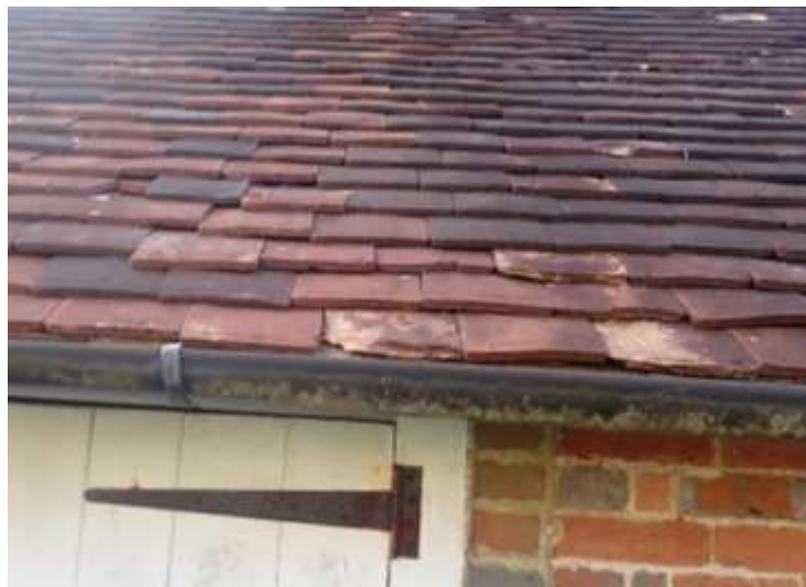
Fig.4 – Uneven clay tiles on roof of outbuilding
