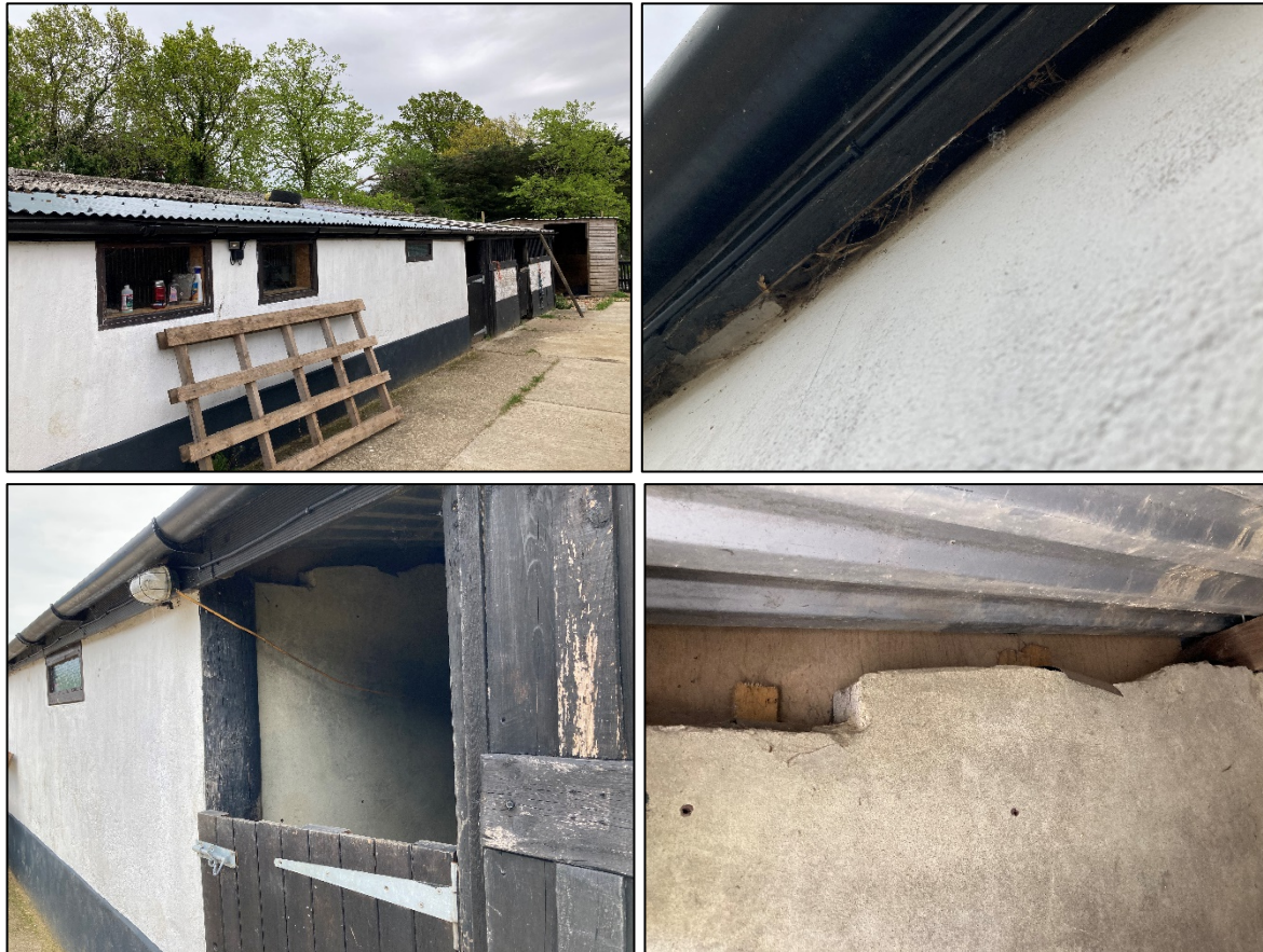
Photograph 5. A view of the western elevation. Note the cobwebbing under the eaves and the large gap between the breezeblock and the roof giving access to a small wall cavity which was heavily cobwebbed.
