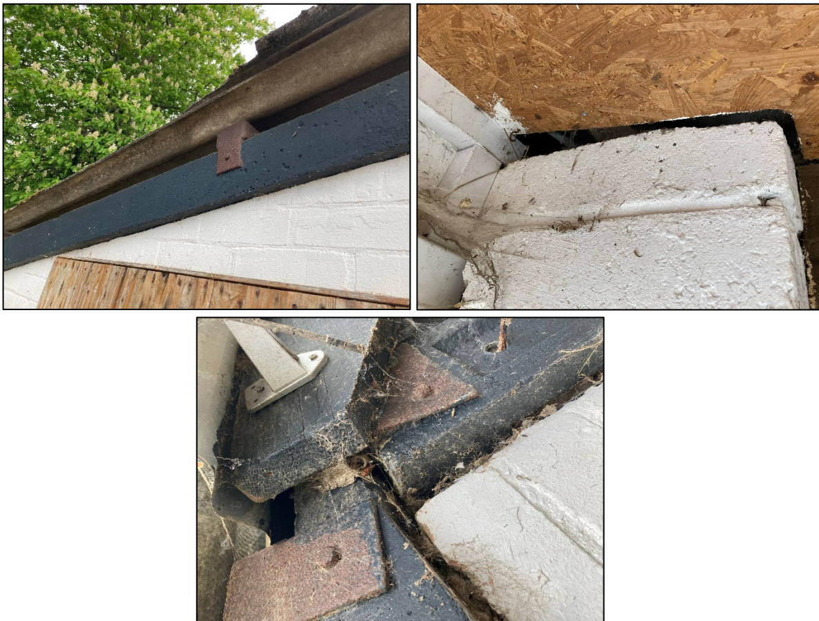
Photograph 2. The gaps suitable for bats on the northern elevation. Note the right and bottom locations were further assessed using an endoscope.
