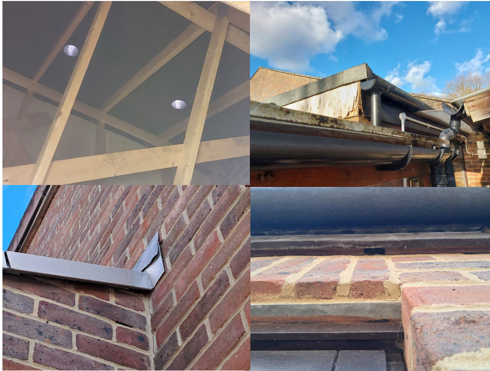
Images 12 - 15: Internal view of roof void of B01, with circular tiles allowing potential ingress into building (top left). Damaged fascia to southeastern aspect (top right). View of gap between wall and metal edge strip (bottom left). View of cavity within fascias of B01.
