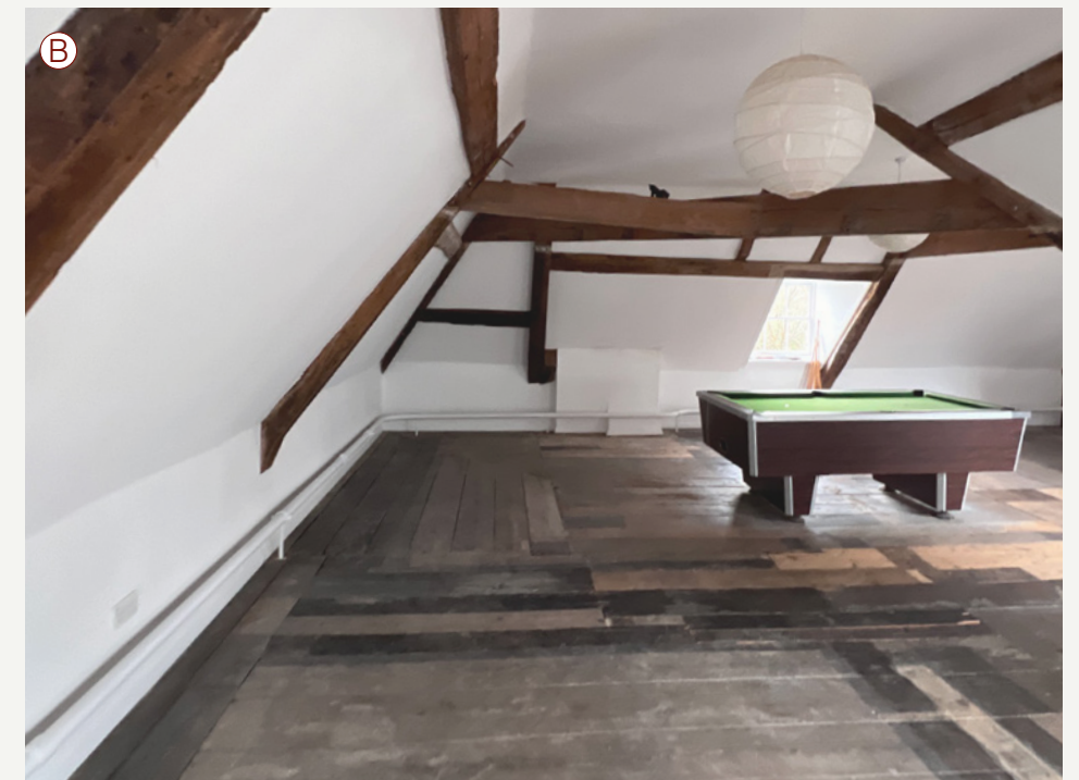
FLOORBOARD DISCOLORATION INDICATES TRACES OF PRE-EXISTING PARTITIONS.
