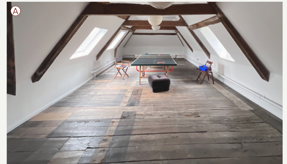
FLOORBOARD DISCOLORATION INDICATES TRACES OF PRE-EXISTING PARTITIONS.
