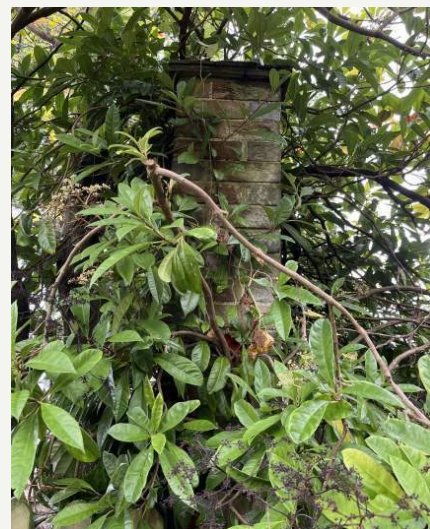
3 Visible excessive lean to wall end, not measured but approx 50-75mm over full height
