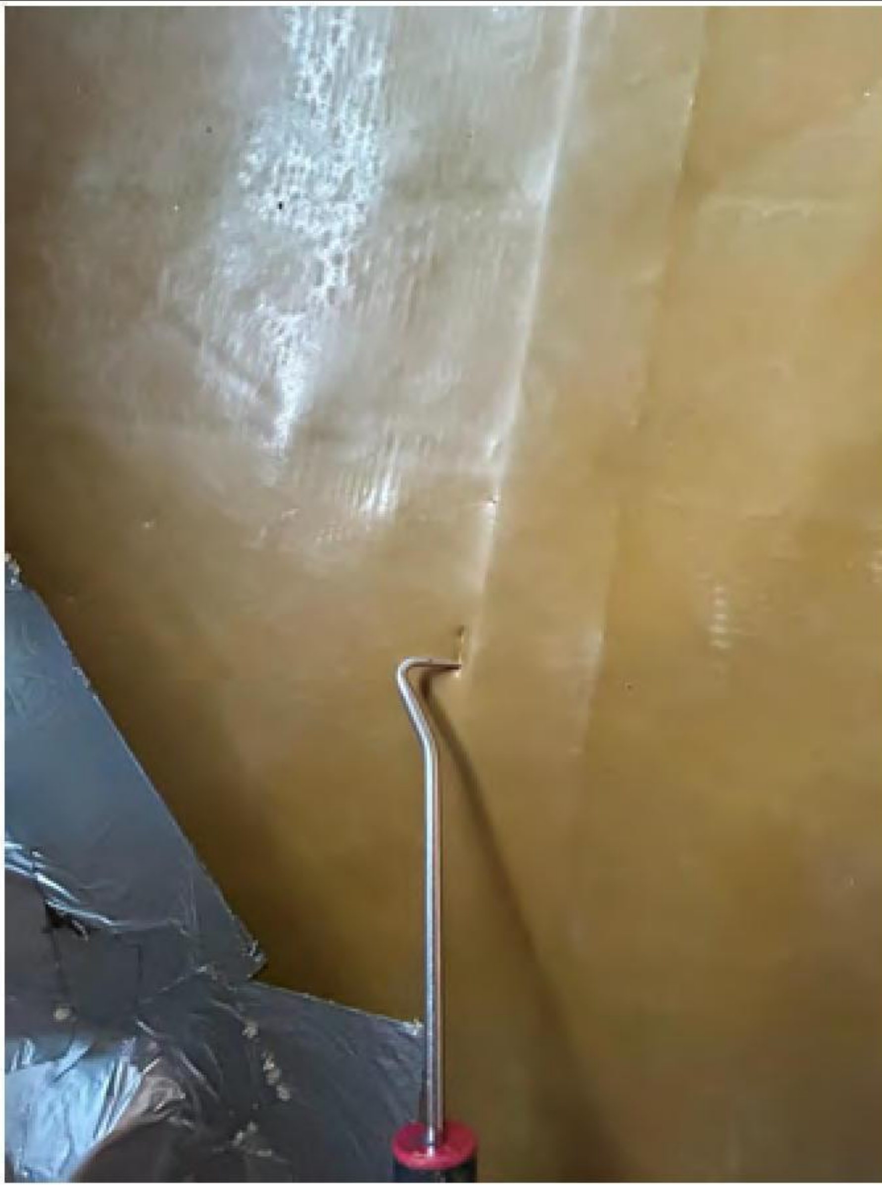
A fault identified.
