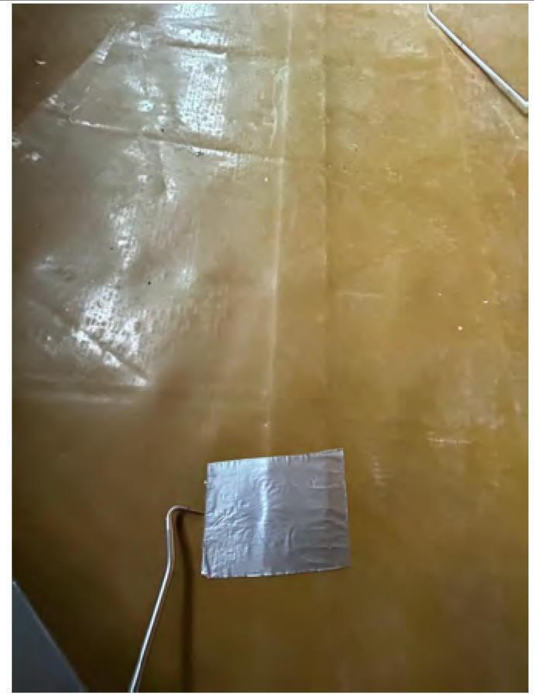
A mechanical point stress test being conducted upon the fault, remediated using Visqueen Pro Detailing Strip.
