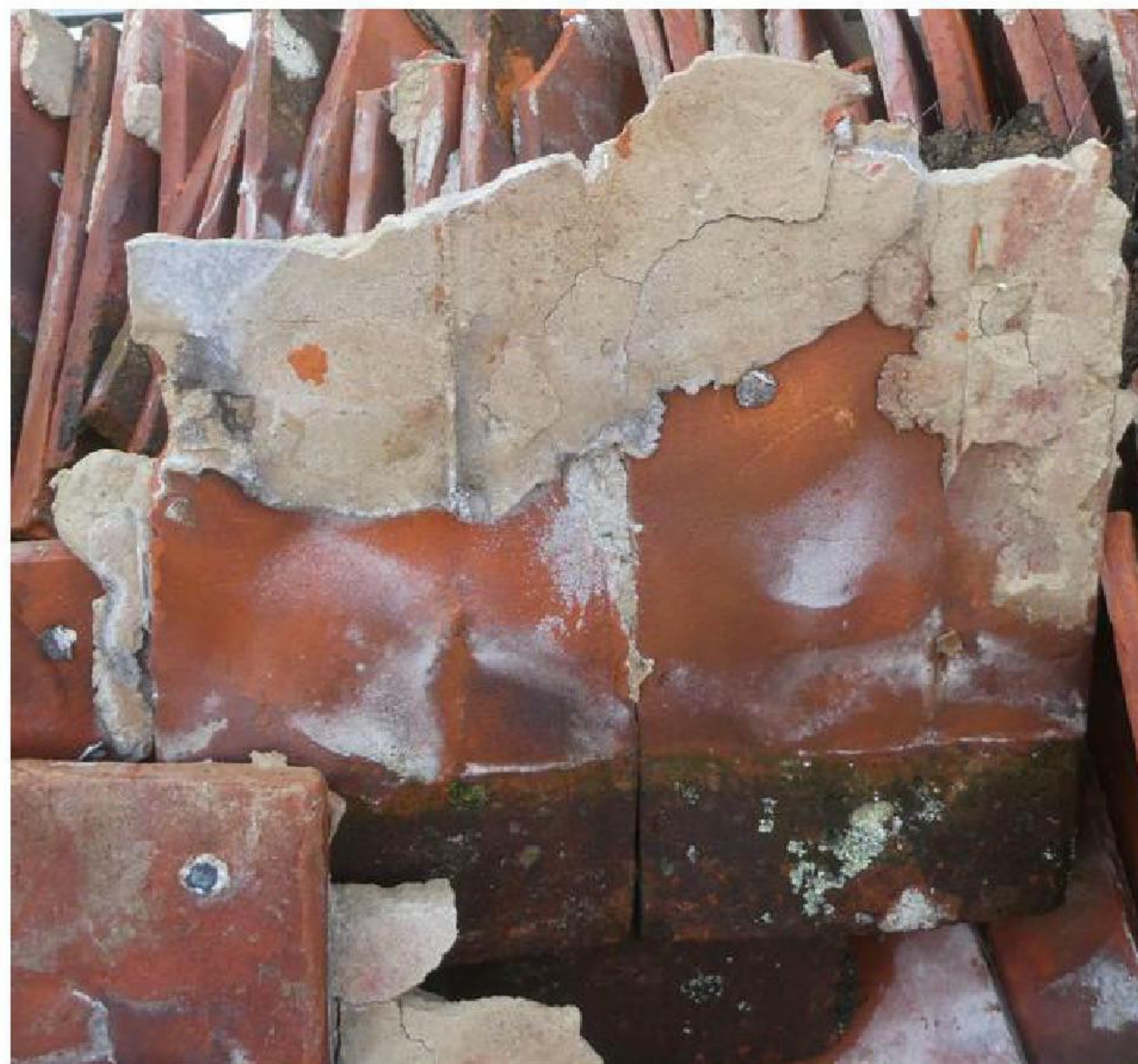
Original tiles with galvanised nails and Portland cement bonding tile together
