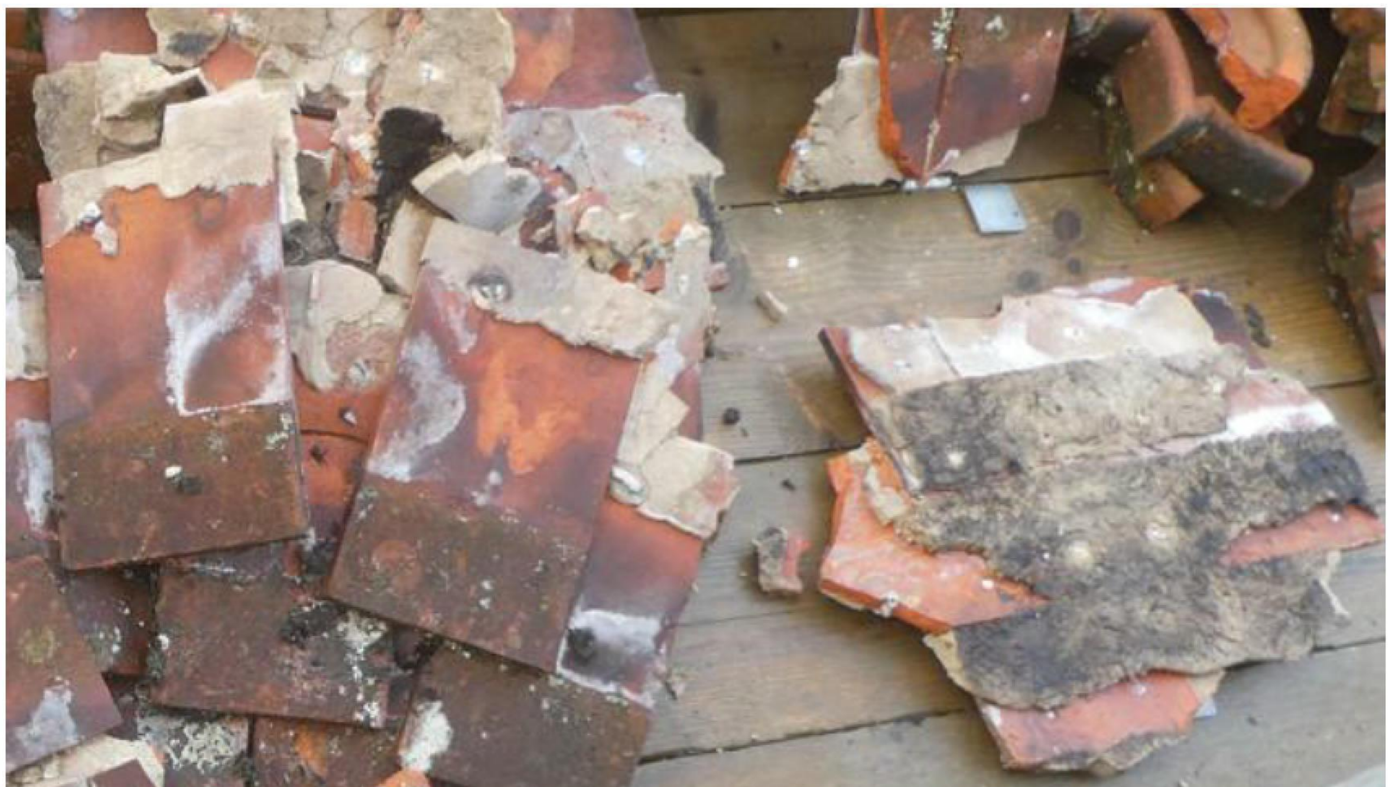
Original tiles cannot be saved due to cement mortar used for bedding
