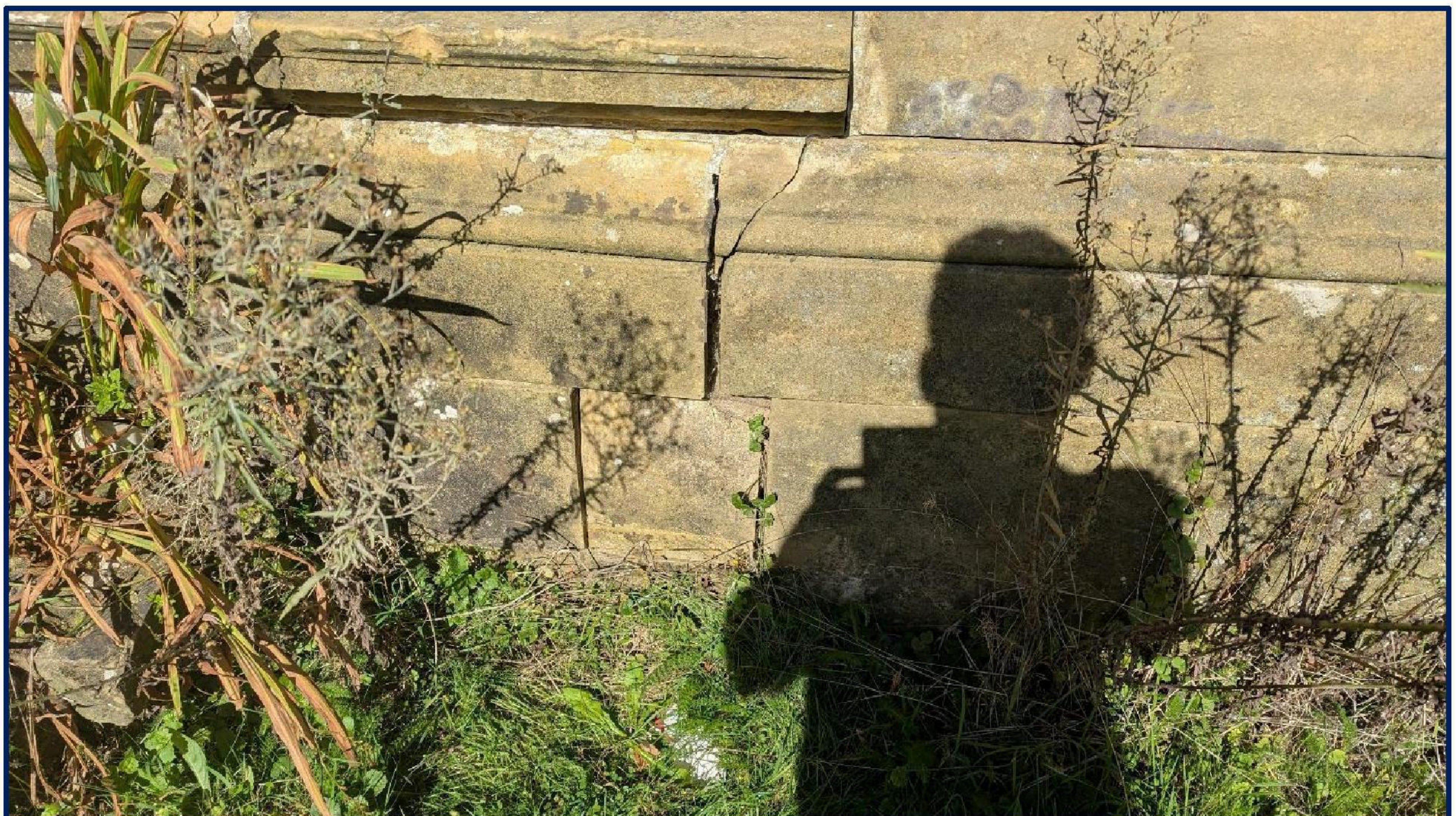
Cracking to the wall
