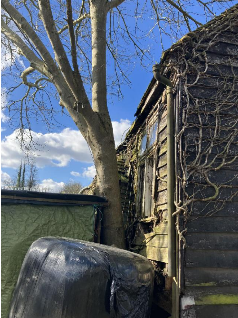
Photograph 1: T29 growing from under the building to be demolished.
