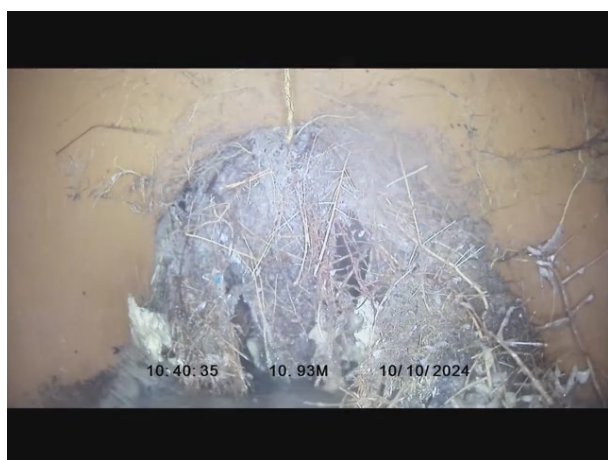
3, 00:00:53, 10.93 m Roots, mass, 80% cross-sectional area loss
