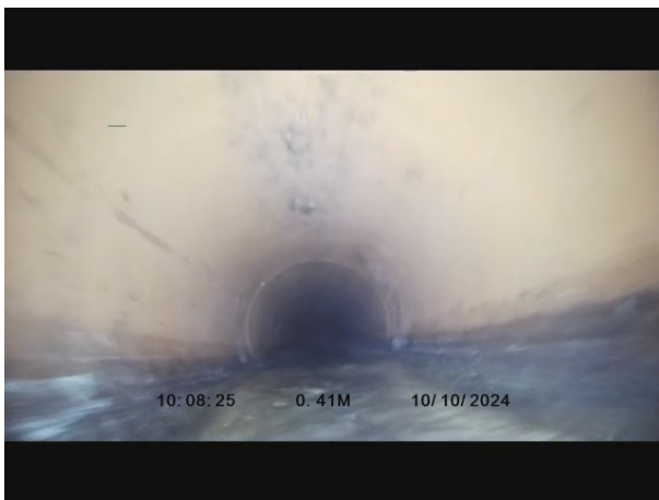
3, 00:00:07, 0.40 m Attached deposits, encrustation from 4 o'clock to 8 o'clock, 5% cross-sectional area loss, start
