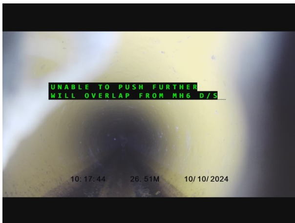
5, 00:03:50, 26.51 m Survey abandoned, Unable To Push Further (Overlap With MH6 Downstream)
