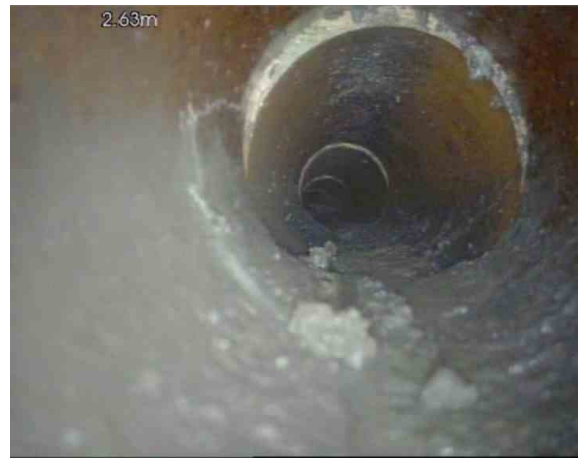
2, 00:00:27, 2.63 m Joint displaced, large
