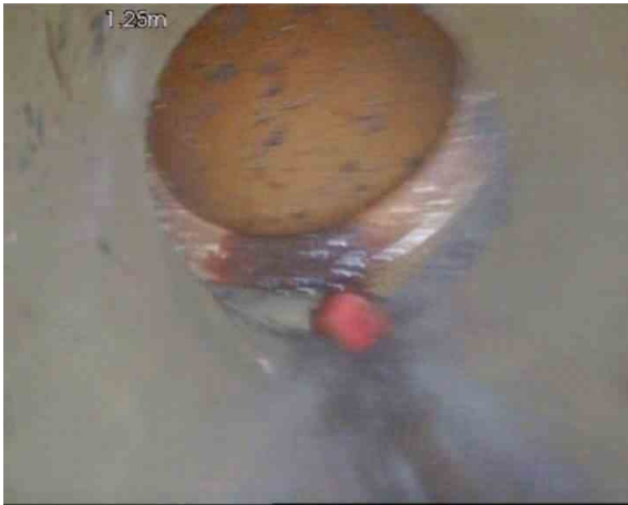
1, 00:00:21, 1.25 m Joint displaced, large
