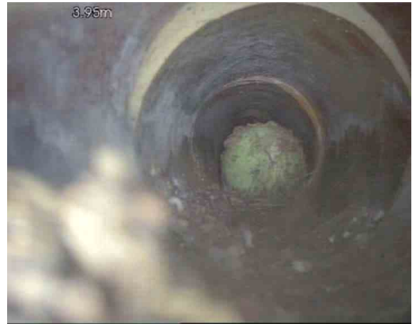
2, 00:00:28, 3.95 m Joint displaced, medium
