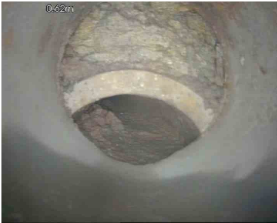
1, 00:00:14, 0.62 m Joint displaced, large
