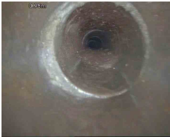
1, 00:00:15, 0.98 m Joint displaced, medium
