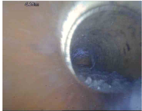
2, 00:00:32, 4.68 m Joint displaced, medium
