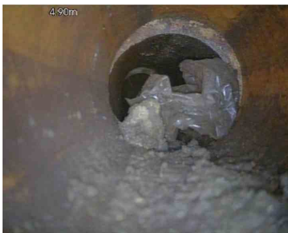
3, 00:00:41, 4.90 m Joint displaced, large
