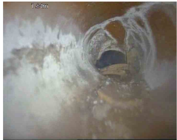
2, 00:00:16, 1.64 m Broken pipe from 5 o'clock to 7 o'clock
