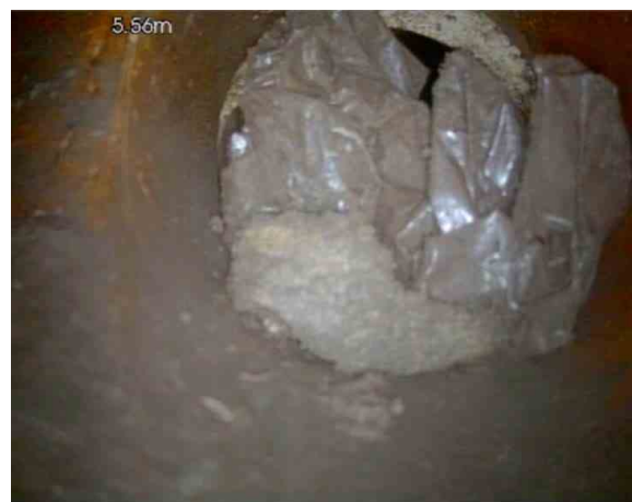
4, 00:01:02, 5.56 m Joint displaced, large
