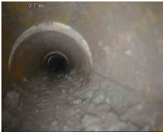
1, 00:00:19, 0.71 m Joint displaced, medium
