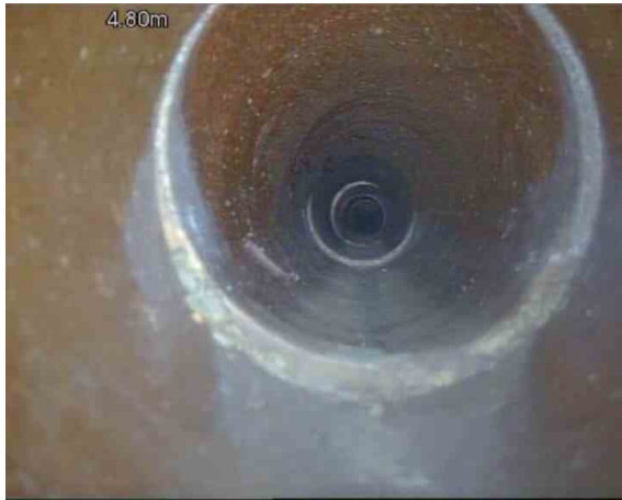
1, 00:00:25, 4.80 m Joint displaced, medium
