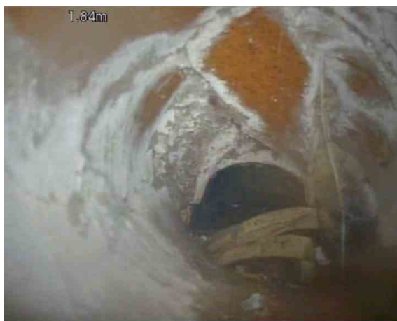
3, 00:00:17, 1.84 m Broken pipe from 9 o'clock to 4 o'clock
