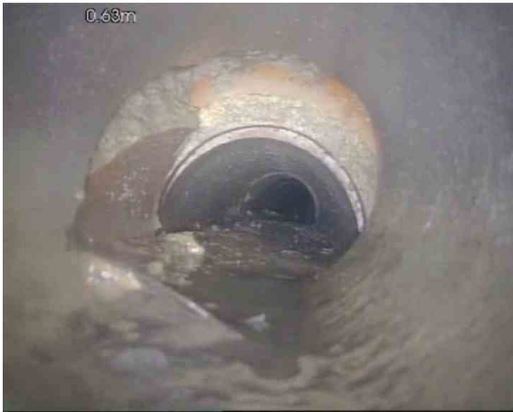
1, 00:00:19, 0.63 m Broken pipe from 8 o'clock to 11 o'clock
