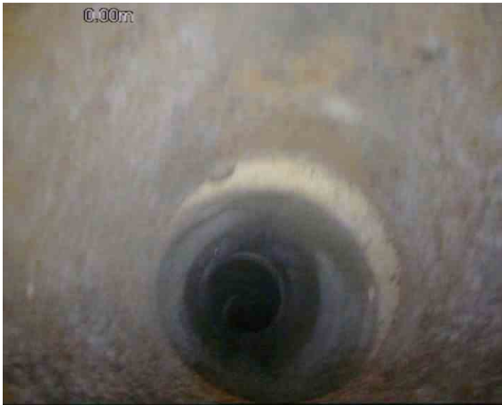
1, 00:00:11, 0.10 m Joint displaced, medium
