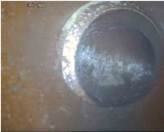
1, 00:00:15, 0.72 m Joint displaced, large
