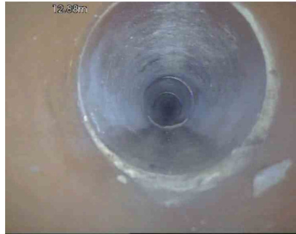
2, 00:00:52, 12.88 m Joint displaced, medium
