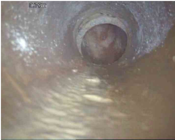
1, 00:00:15, 1.03 m Joint displaced, large
