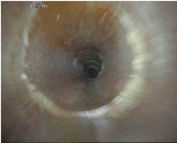
1, 00:00:18, 1.17 m Joint displaced, medium
