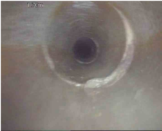
1, 00:00:19, 1.70 m Joint displaced, medium
