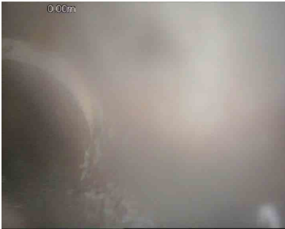
1, 00:00:11, 0.10 m Joint displaced, medium
