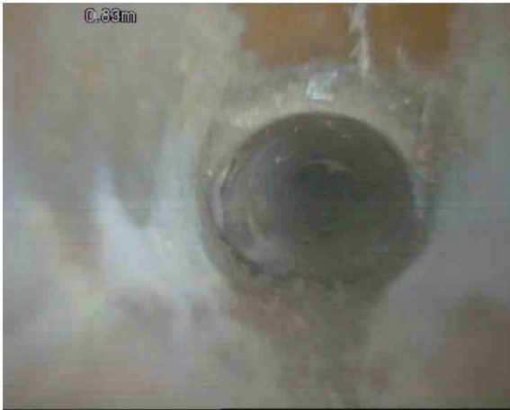
1, 00:00:15, 0.83 m Joint displaced, large
