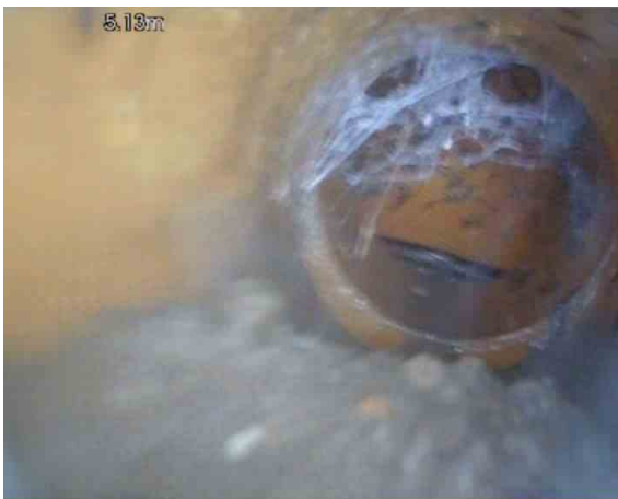
3, 00:00:34, 5.30 m Joint displaced, medium
