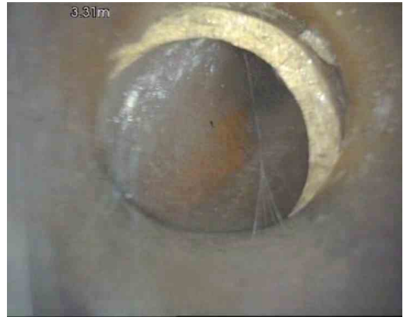
2, 00:00:22, 3.31 m Joint displaced, large
