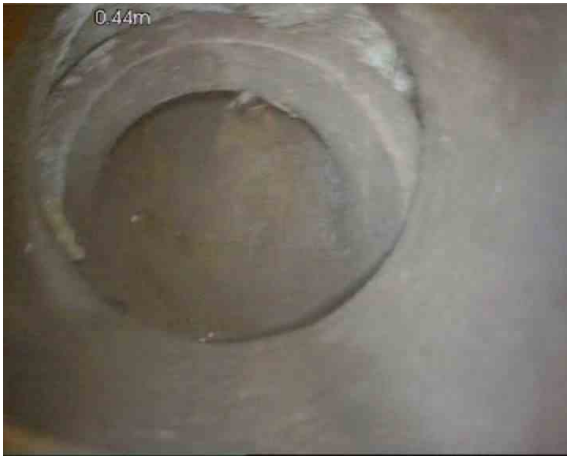
1, 00:00:15, 0.44 m Joint displaced, large
