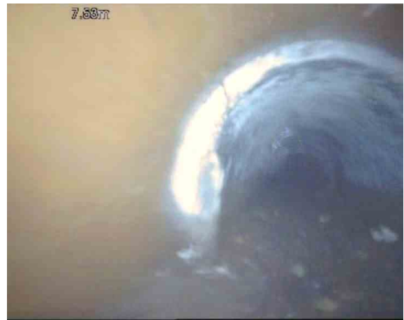
2, 00:00:39, 7.53 m Broken pipe at joint at 10 o'clock
