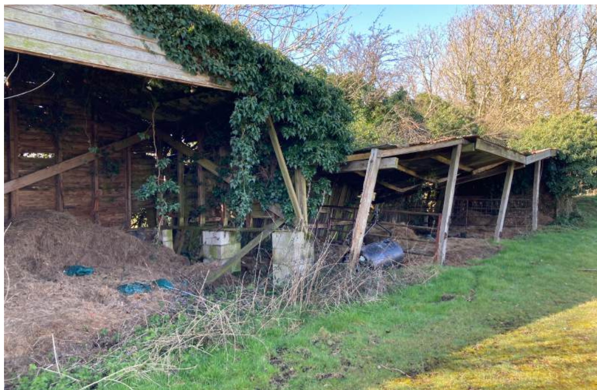
Modern dilapidated buildings to be replaced.
