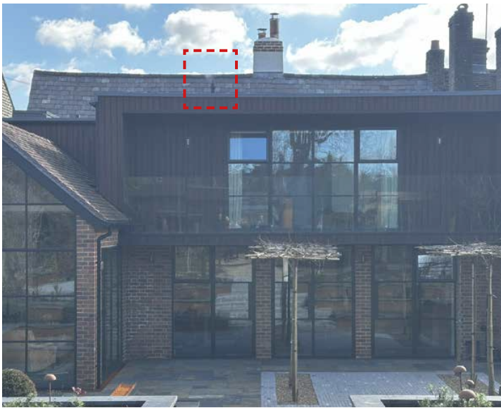
Recent photograph capturing the new boiler flue
