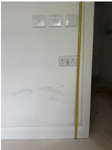
Photo 8 - Example of compliant socket and switch heights
