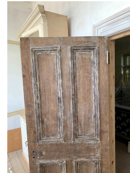
Example of door restoration and decoration required
