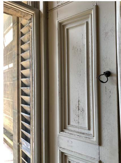
Example of timber shutter requiring restoration
