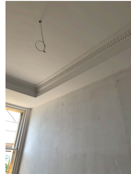
Example of ventilation dropped ceiling with cornicing
