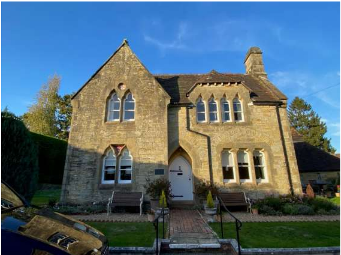
Figure 19: Damaged, missing or broken crested ridge tiles to the principal south elevation
