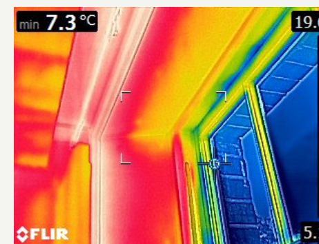
82 Limited thermal bridge around window. Air ingress to perimeter of sash.
