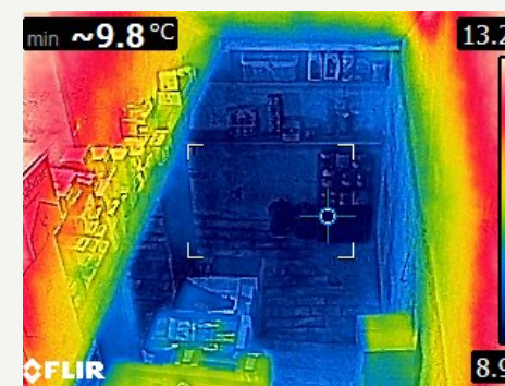
135 Temperature change below ground floor level evident.
