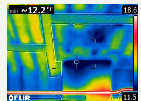
266 Very poor levels of insulation to vertical surfaces. Chimney is a significant thermal bridge where it passes through the roof. Evidence of damp in chimney breast. Likely to be condensation as often below dew point.
