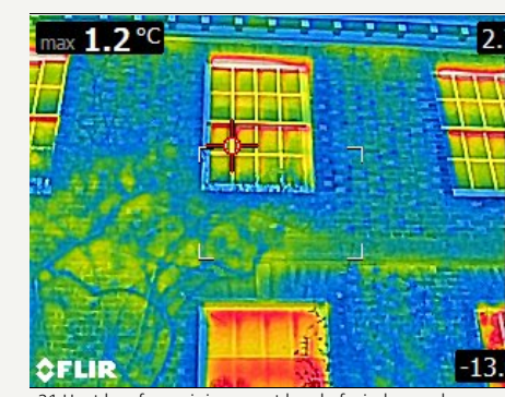
21 Heat loss from air ingress at head of window and horizontal sash junction.
