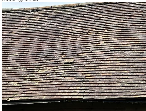
B9 Barn – example of lifted, missing or broken tiles common across the roof
