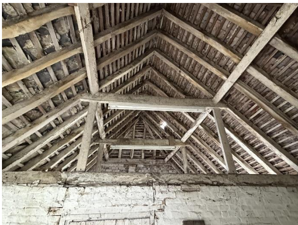
B2 Dairy – internal roof structure with crevices behind timbers
