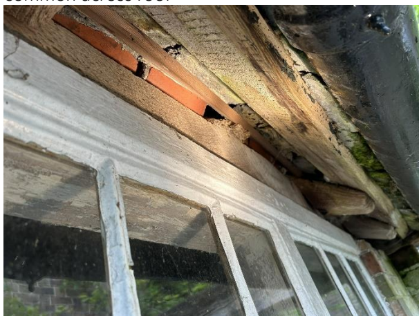
B2 Dairy – example of gaps at eaves
