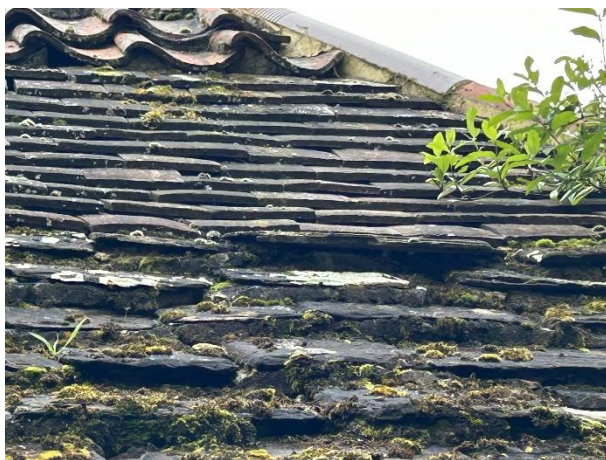
B2 Dairy – example of lifted and missing tiles common across roof
