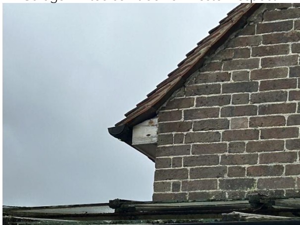
B4 Garage – gap at box end on north-eastern corner
