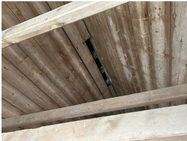
B4 Garage – example of internal missing panelling
