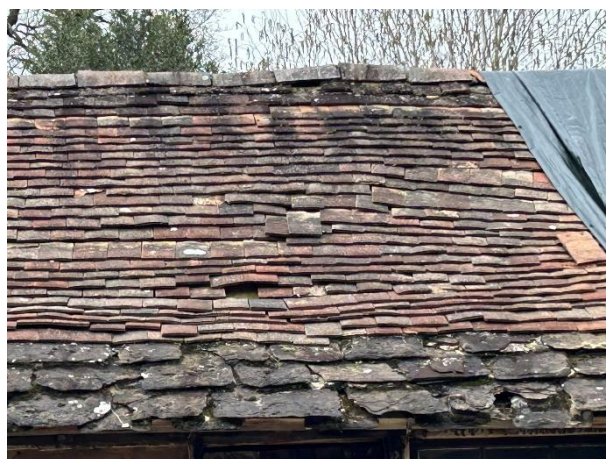
B7 Cowshed – example of missing, lifted or broken tiles that are extensive across the roof
