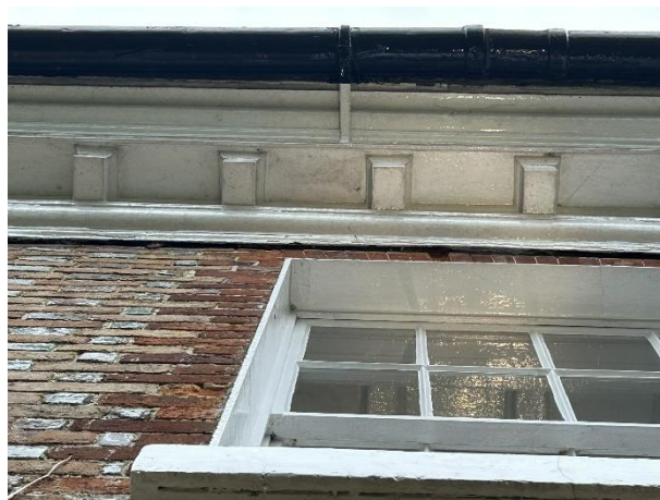
B1 Main House –lifted soffit on western aspect
