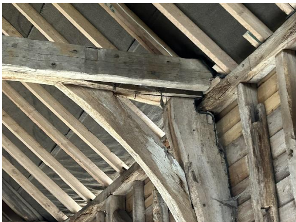
B9 Barn – internal roof structure with crevices at timber joints
