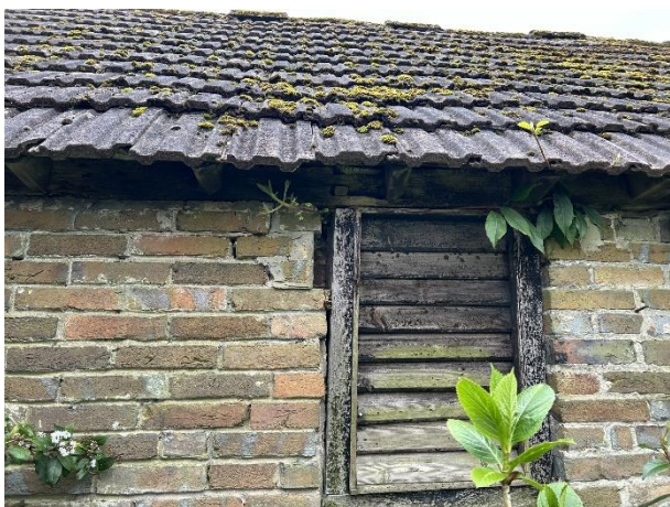
B6 Stable – shutters and broken brickwork at northern aspect
