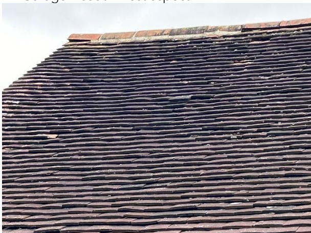
B4 Garage – lifted and missing roof and ridge tiles on western aspect
