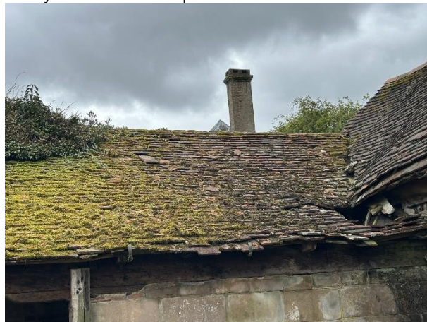
B8 Byre – example of lifted, missing and broken roof tiles
