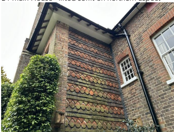
B1 Main House – lifted hanging tiles on northern aspect
