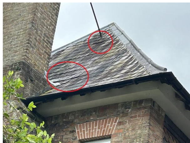
B1 Main House – example of lifted tiles common across roof
