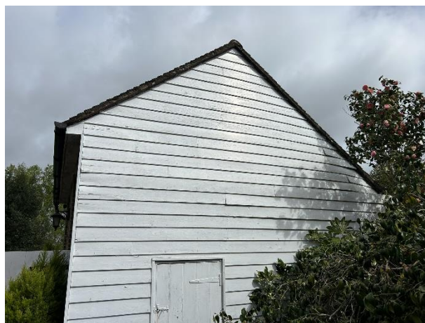
B3 Log shed – broken panelling on southern aspect
