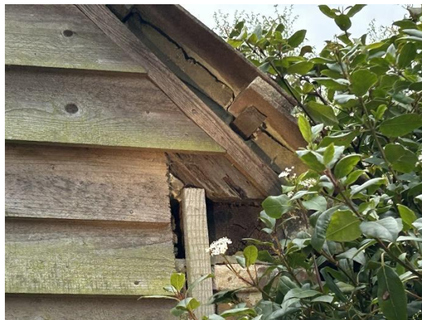
B6 Stable – gaps in timber panelling at eastern aspect
