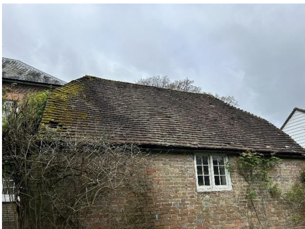
B2 Dairy – example of missing tiles common across roof
