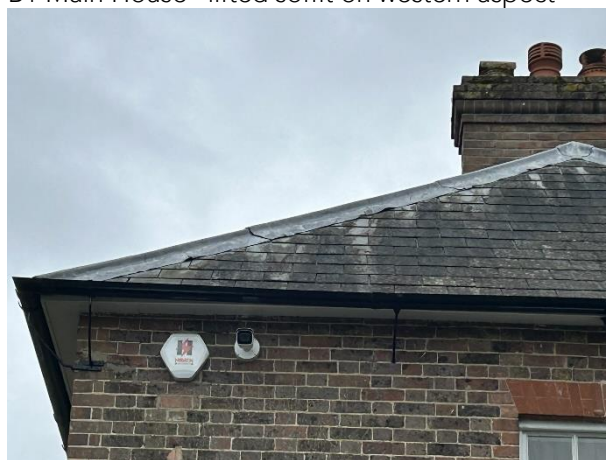
B1 Main House – example of lifted lead flashing
