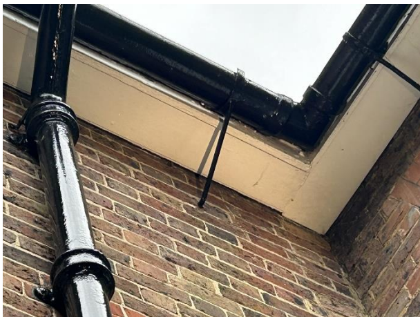
B1 Main House –lifted soffit on northern aspect
