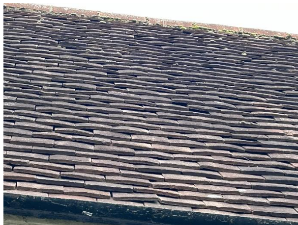
B5 Cottage – example of lifted or missing roof tiles common across the building
