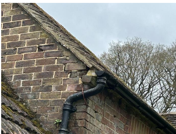
B5 Cottage – broken brick work at north-eastern corner
