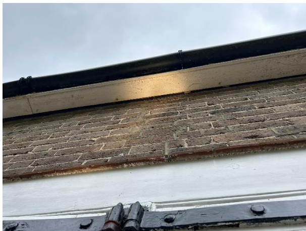
B4 Garage – lifted soffit box on western aspect
