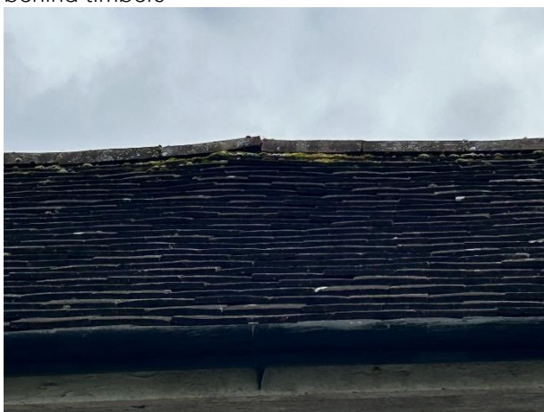
B3 Log shed – lifted tiles and lifted ridge tile on western aspect
