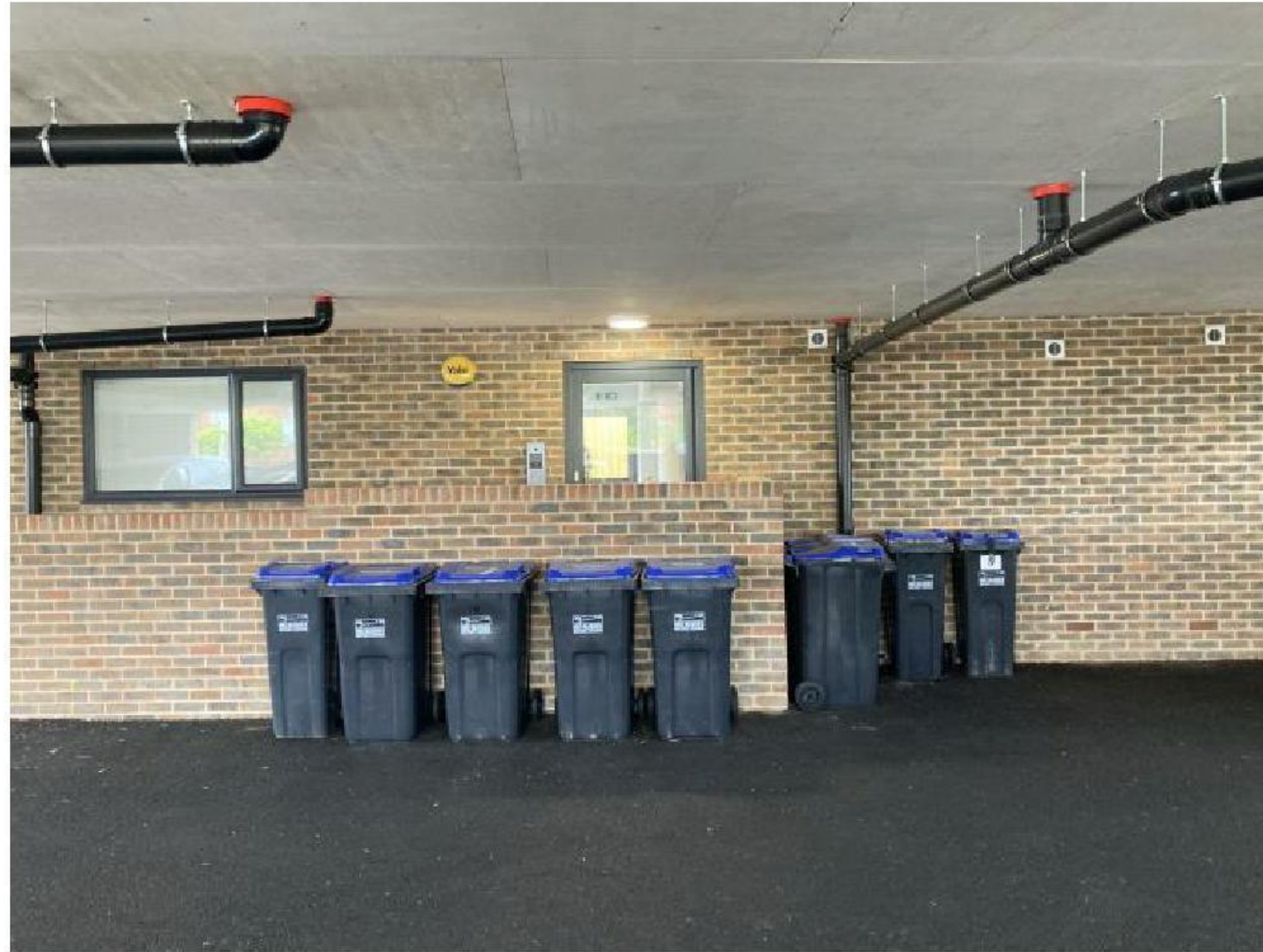
Nine Recycling bins kept within the undercroft
