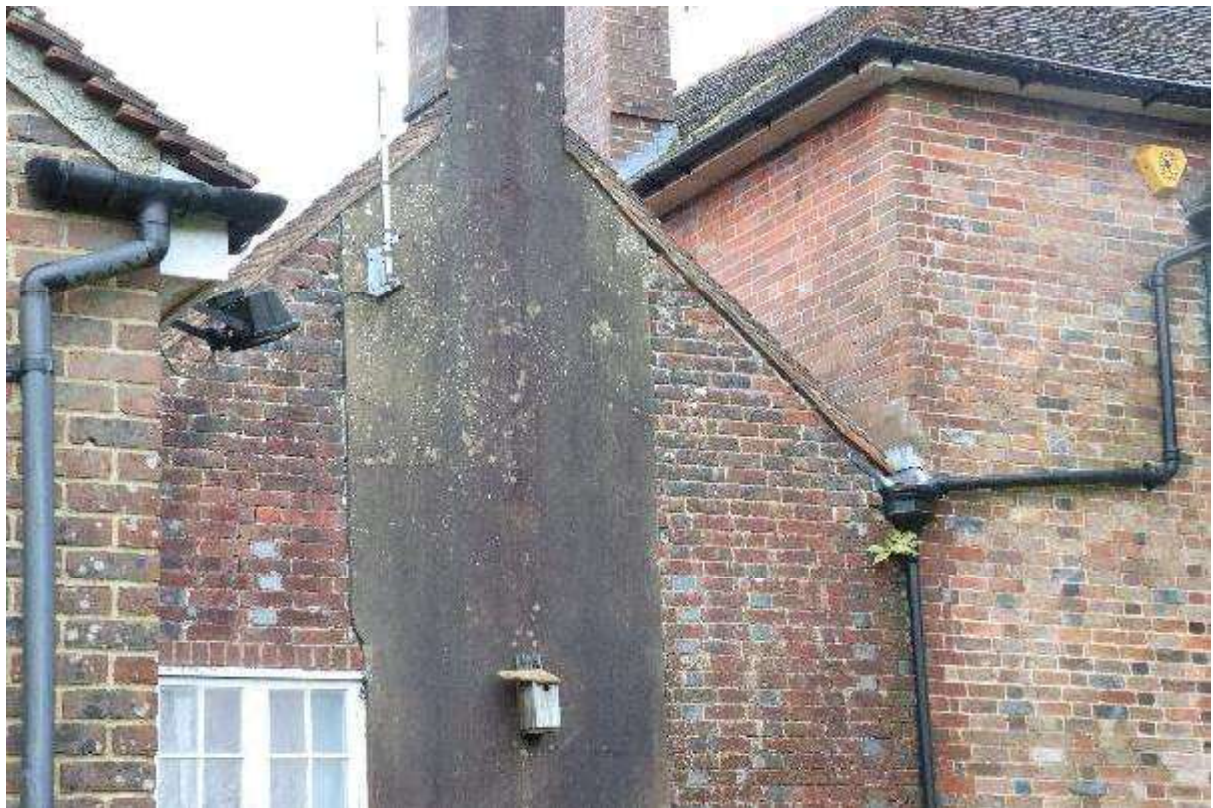
4. Rear Elevation crack detail
