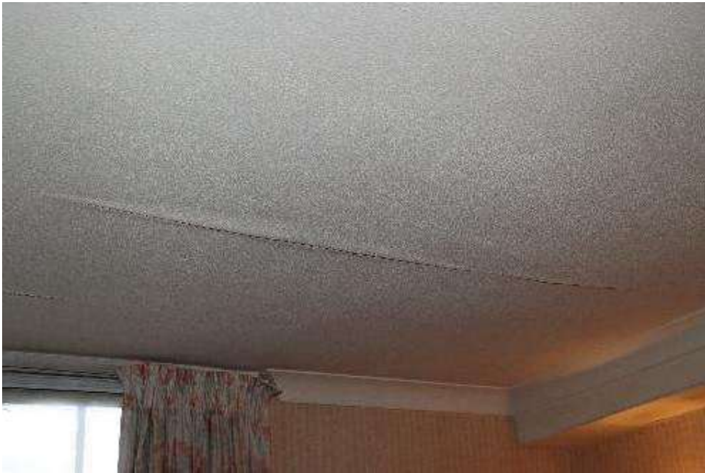
12. Ceiling cover delamination
