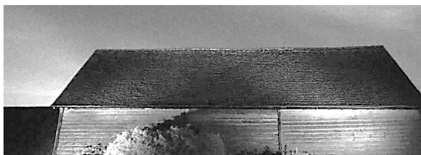
Fig. 15 – Infra-red camera view of E side of barn
