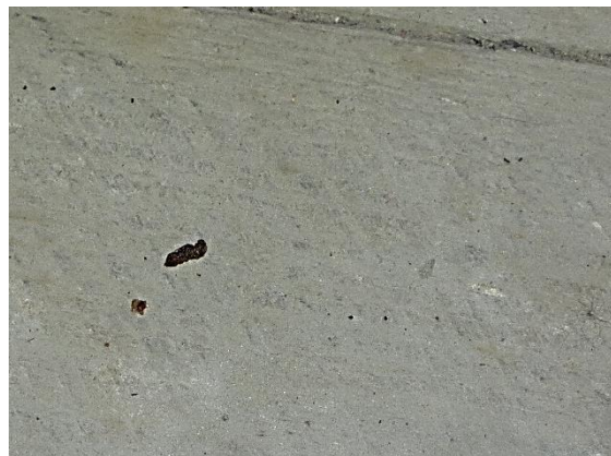
Fig. 12 – bat dropping on floor of mezzanine
