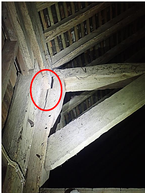
Fig. 11 – Crevices in old timber frame, circled
