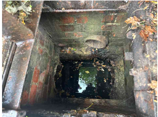
2, 0.00 m Start node, gully, reference: RG
