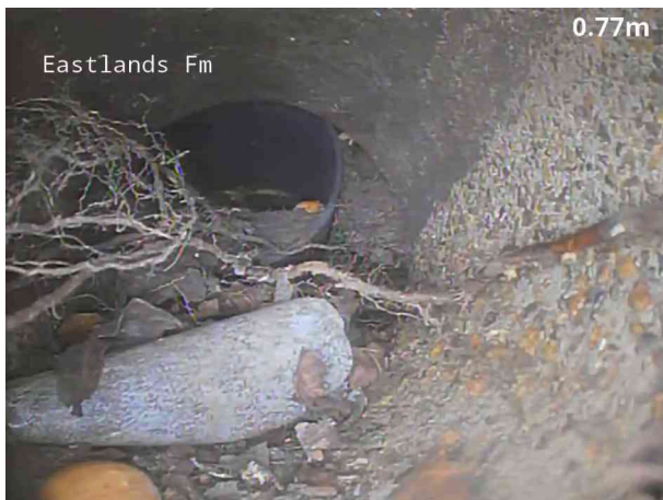
5, 00:00:33, 0.90 m Settled deposits, coarse, 20% cross-sectional area loss
