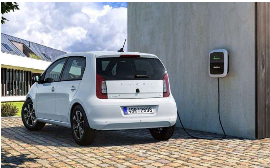
Electric Charging Points
