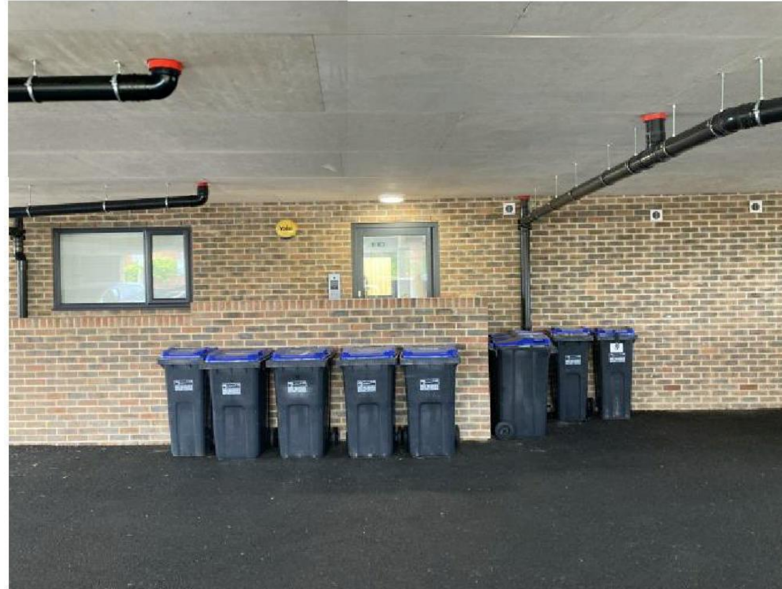
Nine Recycling bins kept within the undercroft
