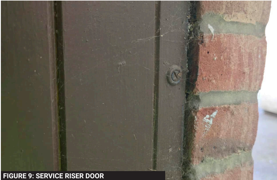
FIGURE 9: SERVICE RISER DOOR
