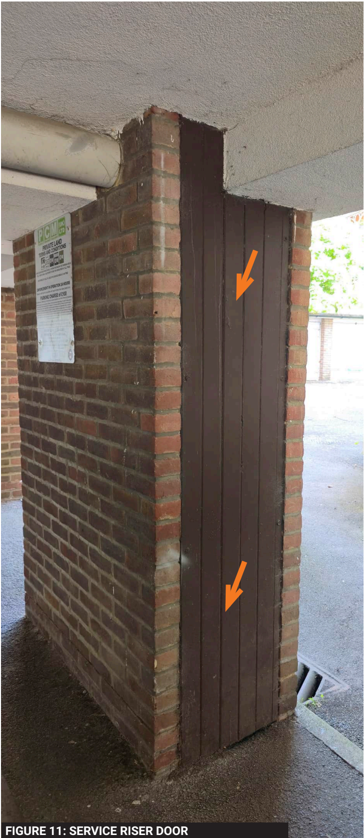
FIGURE 11: SERVICE RISER DOOR
