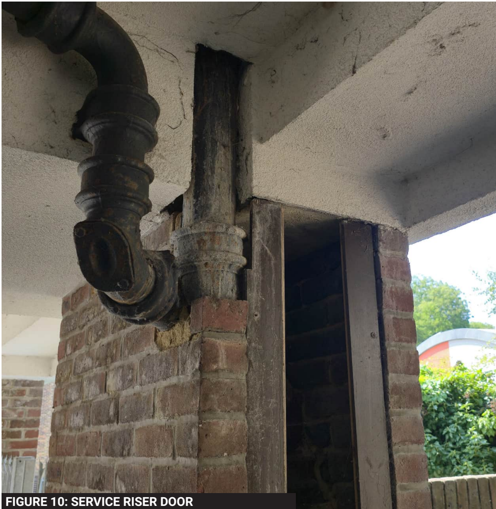
FIGURE 10: SERVICE RISER DOOR
