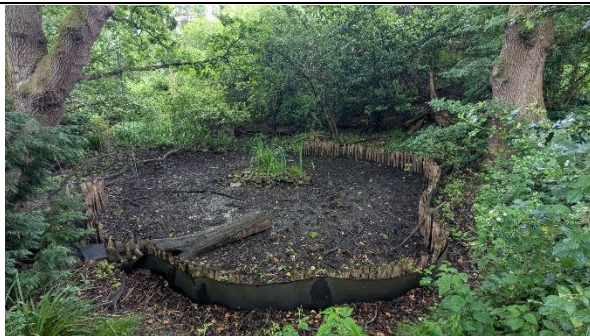
Photo 7: The northern pond as marked has drained due to a perforated lining.
