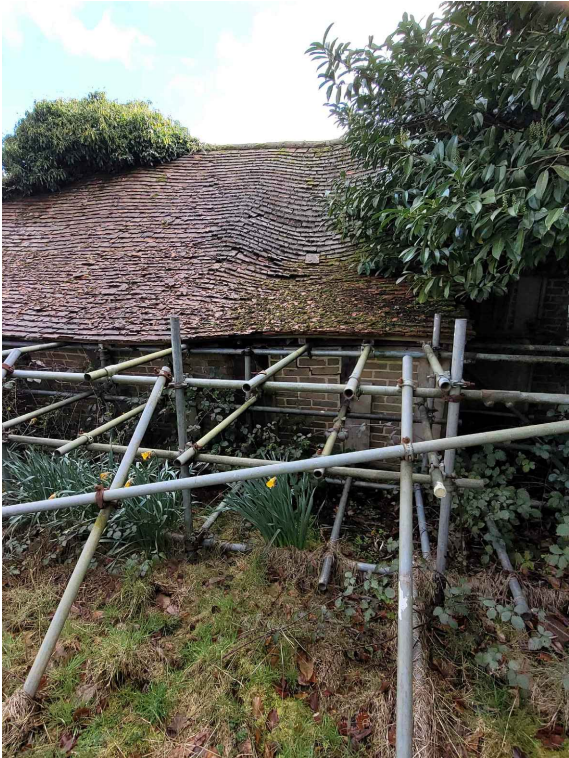
LEANING & CRACKED BRICKWORK DUE TO BROKEN PURLING AND RAFTERS
