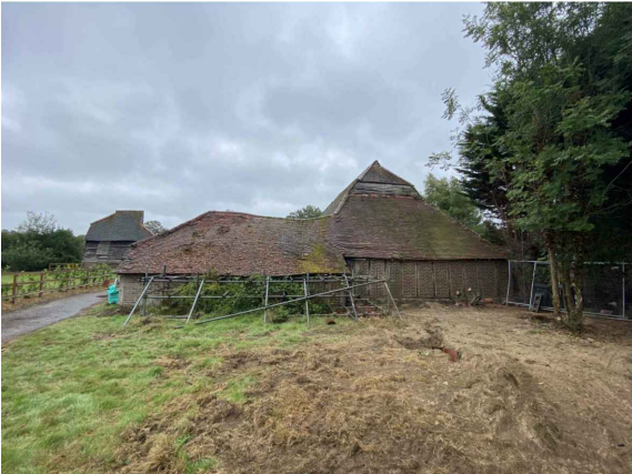
SCAFFOLD HOLDING UP LEANING WALL TO OUTSHOT
