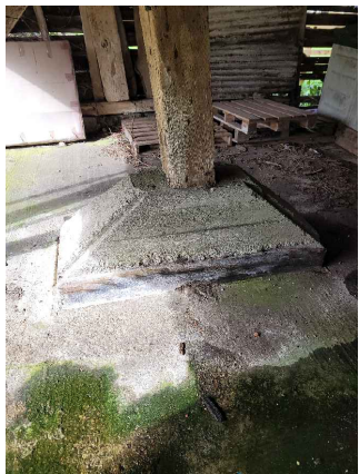
GROUND FLOOR POST
