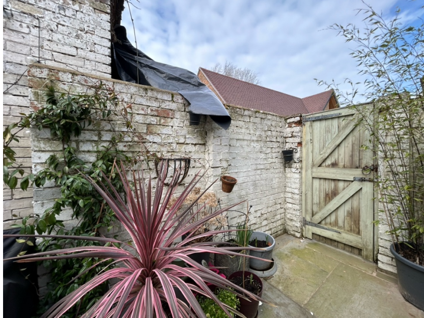
IMAGE 2: The two existing walls of Wyncote in a very poor condition (viewed from within the garden of Wyncote)
