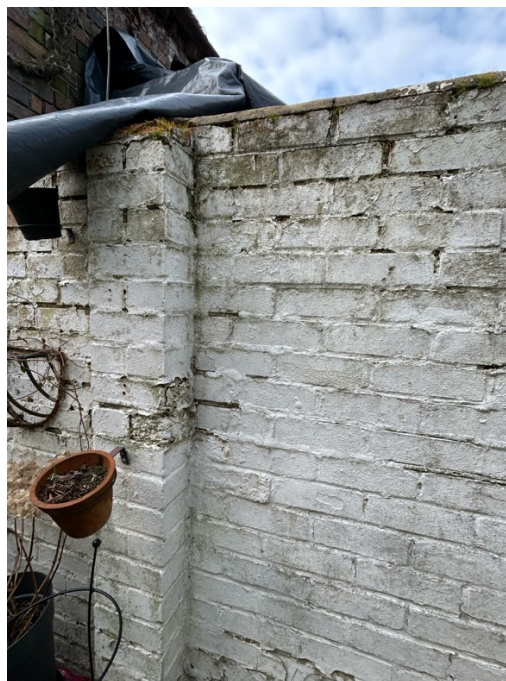
IMAGE 3 – 6 – The condition of the West Wall of Wyncote
