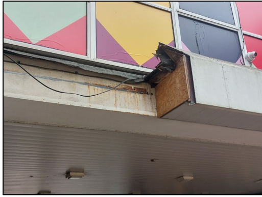
Figure 3: Building 10 showing evidence of deterioration
