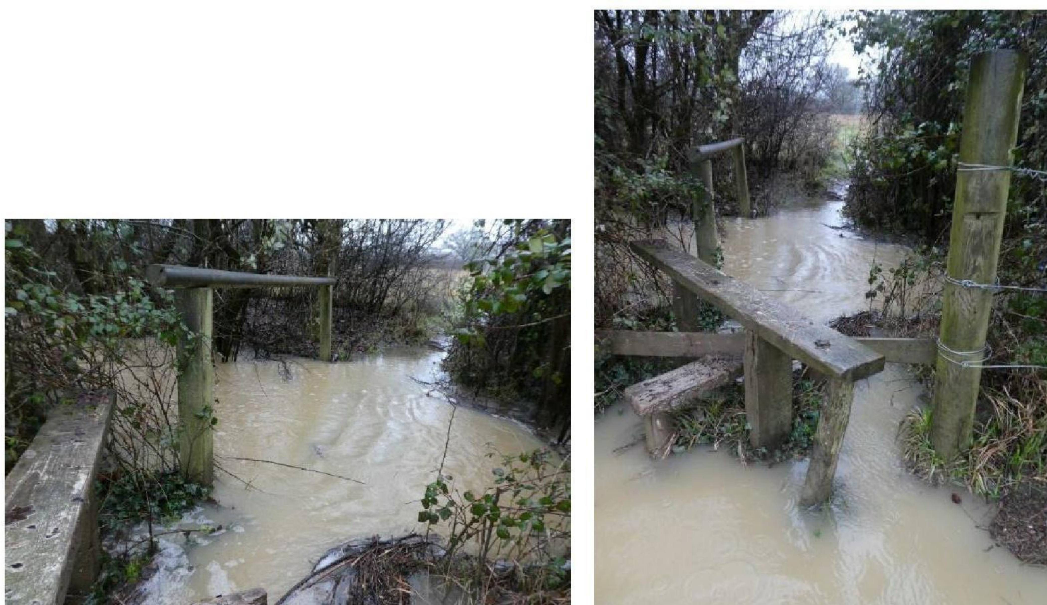
Photographs taken 27/01/2026 at 11am from the western boundary of the site looking west over towards the next field. These are of the footbridge which takes footpath 1AL over the watercourse. That bridge was completely submerged and too dangerous to cross and use. The floodwater level by the stile was nearly 40cm.
