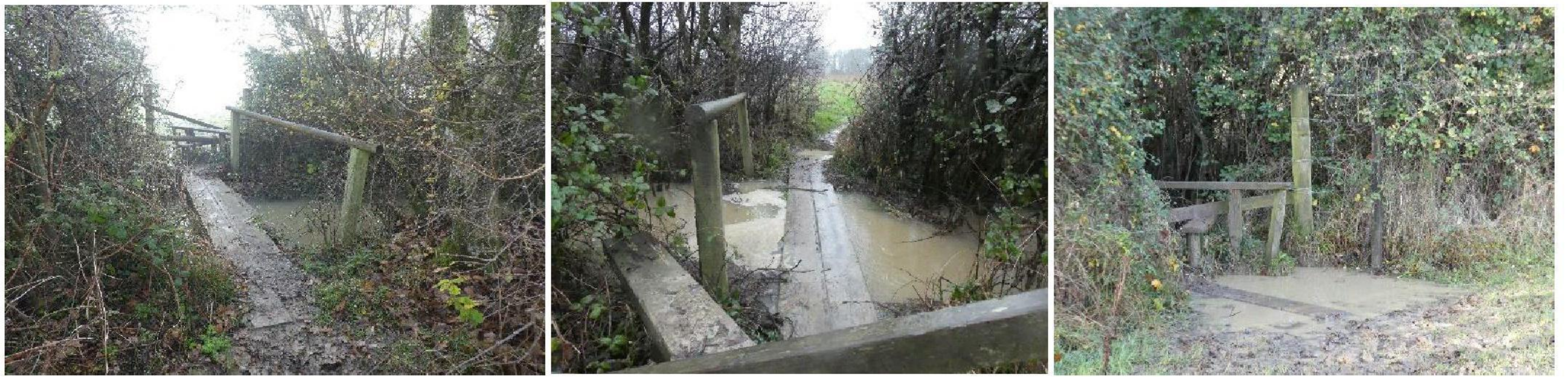
These photographs show what the footbridge looks like when not submerged .Flooding at this point of the site is a regular occurrence. From left to right the photographs were taken on 28/1/2024 at 11am, 05/01/2025 at 3pm and 19/12/2025 at 12pm
