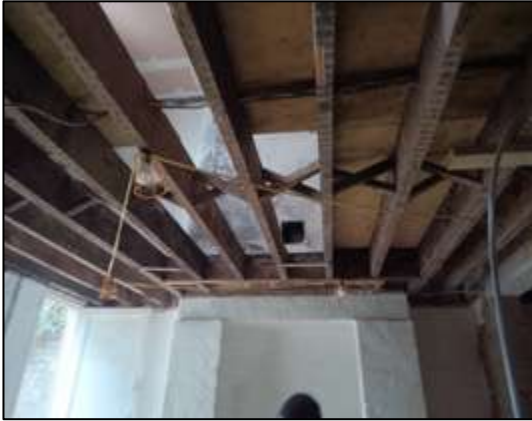
Photograph 7: Missing flooring above the basement allowing access into the main building from basement level.
