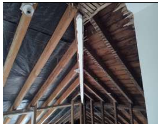
Photograph 12: Stripped ceiling within the roof void of building B1 exhibiting both lined and unlined areas of roof.
