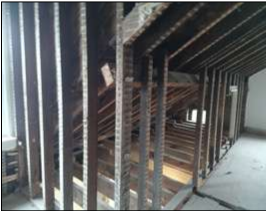
Photograph 9: Stripped back ceilings and floor within the roof void of building B1.
