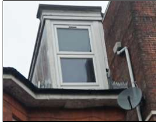
Photograph 2: Dormer on the eastern elevation exhibiting a missing piece of panelling.
