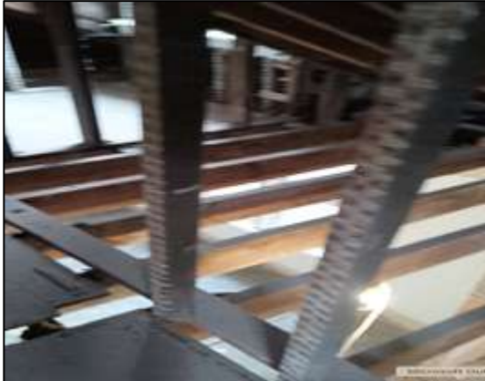
Photograph 13: Missing flooring in the roof void of building B1.
