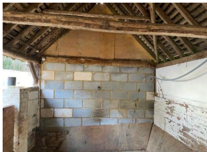
Interior of B3. The roof is unlined. The western wall and southern gable end are boarded, creating potential crevice features accessed by the warped/rotten external weatherboarding.
