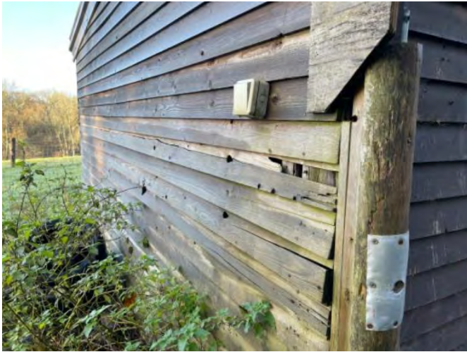
Damaged weatherboarding on the southern end of B6, with potential crevice features.
