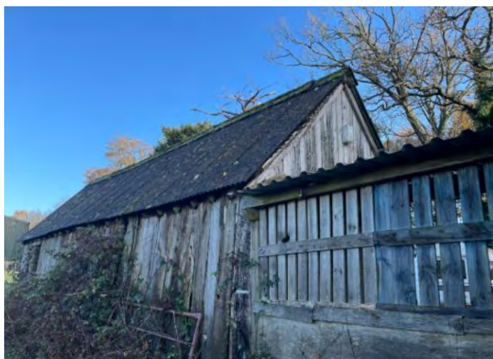
Western elevation and southern gable end of B3 with warped and rotten timber, creating potential crevice roosting features.
