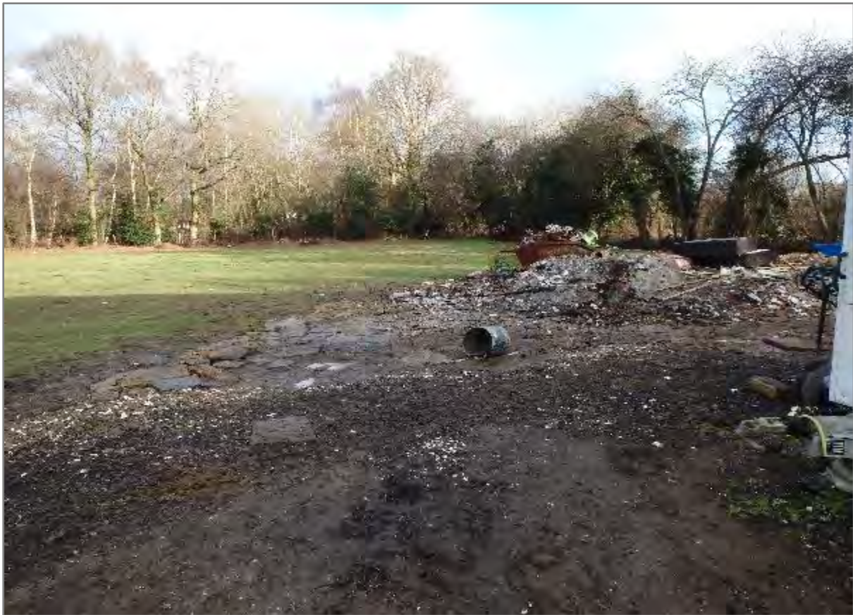
Plate 8: Concrete flooring and rubble located to the north of the barns in the western part of the Site (looking N).
