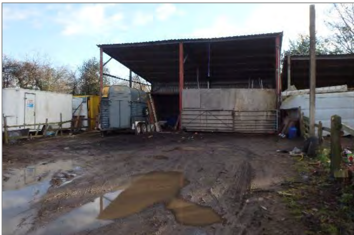
Plate 4: First shed/barn in the west of Site at the eastern end of the trackway (looking E).
